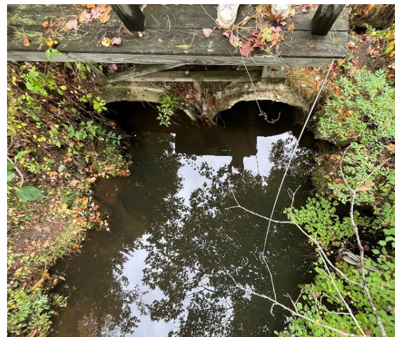
Pond A Outfall
