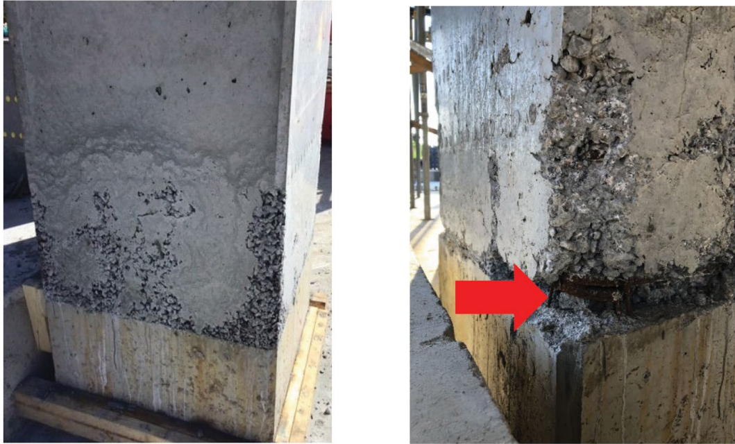
Figure 13. Honeycombing in New Concrete and Honeycombing with Exposed Rebar Source: USACE Savannah District.
