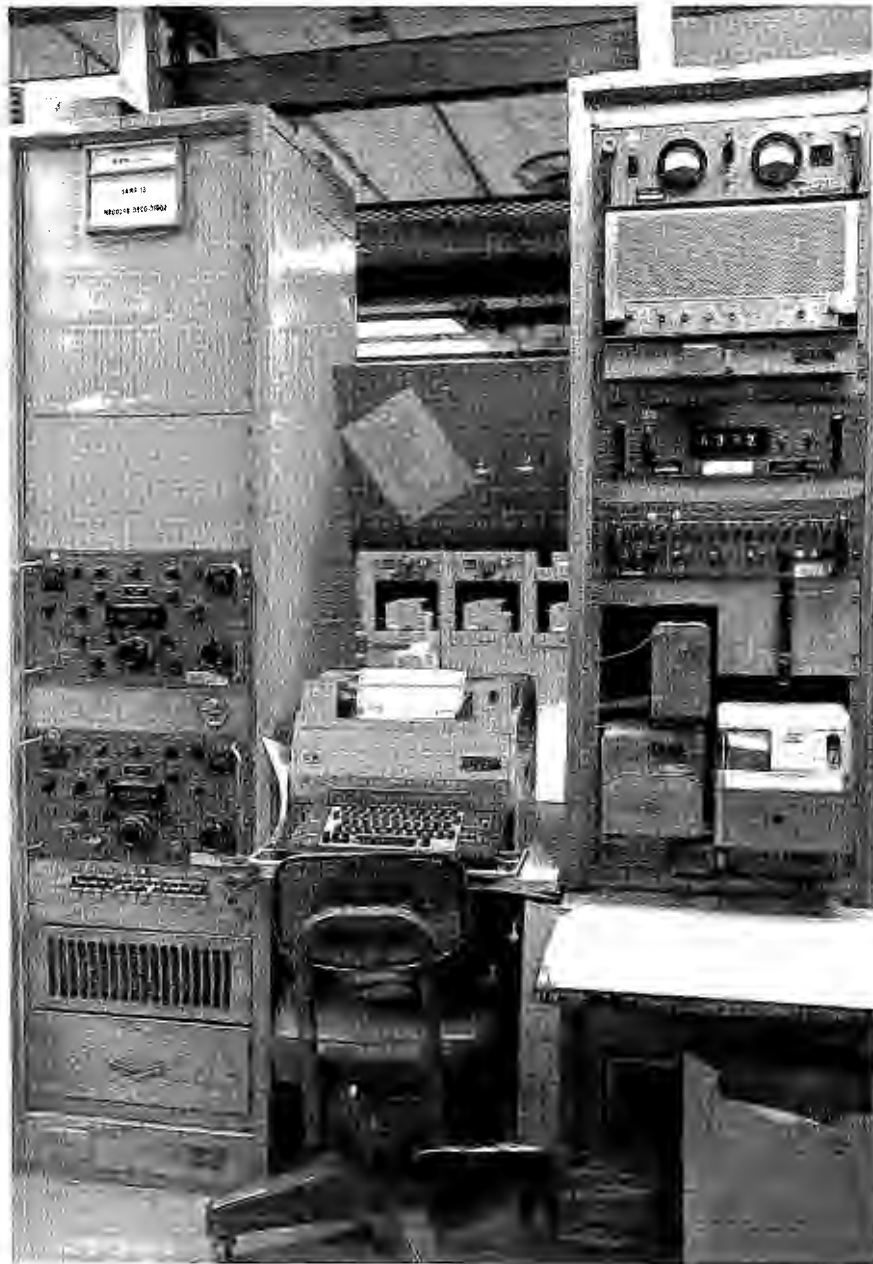
AG-22 - Configured Morse Position at [redacted] (R-390 receivers are in the left-hand rack; MOD-35 in the center; and tape unit on the right)
