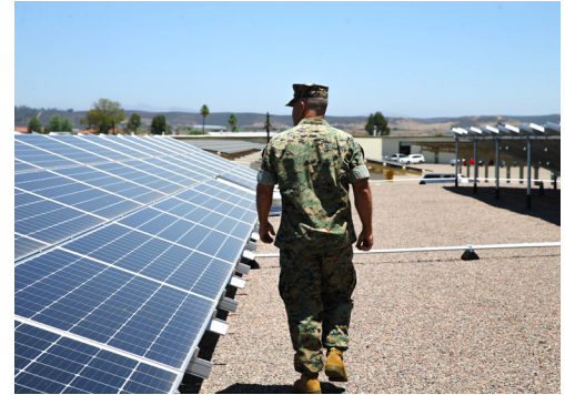
Director of Technology and Partnerships for the Marine Corps Installation Next Program observes solar panels at Marine Corps Air Station Miramar on July 15, 2020.
