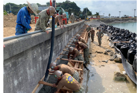
Navy Seabees deployed with Naval Mobile Construction Battalion (NMCB) 5 place concrete for the seawall project on board White Beach Naval Facility. NMCB-5 is deployed across the Indo-Pacific region conducting high-quality construction to support U.S. and partner nations to strengthen partnerships, deter aggression, and enable expeditionary logistics and naval power projection.
