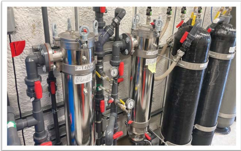
Site 5 PFAS Pilot Test Filtration System Source: Tetra Tech
