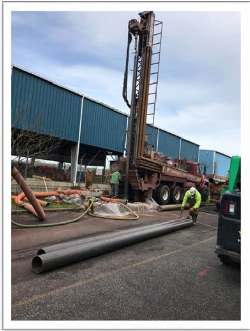
Example of Monitoring Well Installation: Wells are used to sample groundwater. Source: Tetra Tech
