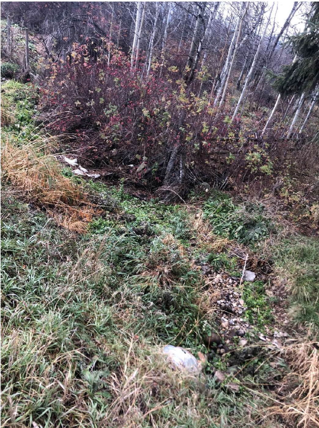
Photo 8. Culvert Outlet and channel on West side of Highway 33. Taken from Photo Point 3.
