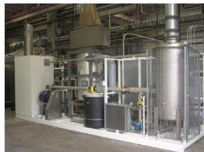
One 3 GPM (11.3 LPM) iSCWO skid
