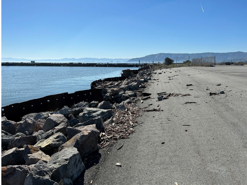
Parcel D-1 Photograph 17: Shoreline revetment east of Building 381. Facing southeast. Photographed by: Marcella Navas/CH2M, 2/9/2023
