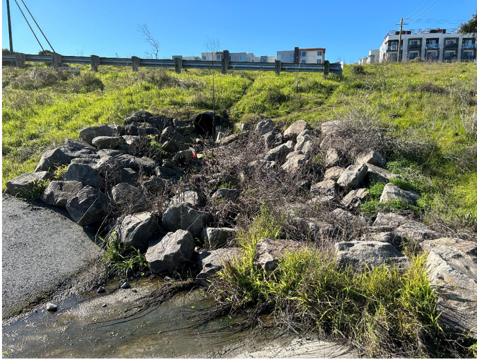
Parcel B-1 Photograph 3: Outfall protection for storm drainpipe southwest of Building 120. Facing southwest.
