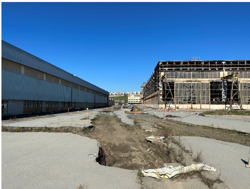
Parcel G Photograph 10: Excavation west of Building 411 and east of Building 439. Facing northwest. Photographed by: Marcella Navas/CH2M, 2/9/2023
