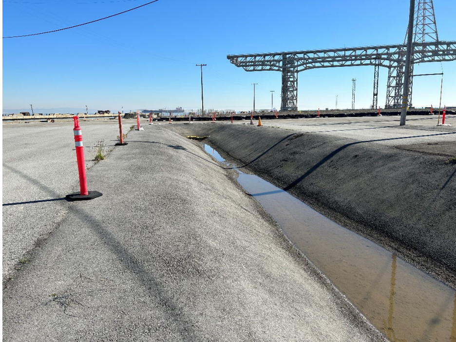
Parcel D-1 Photograph 9: Drainage swale with water southeast to Building 307. Facing northeast.
