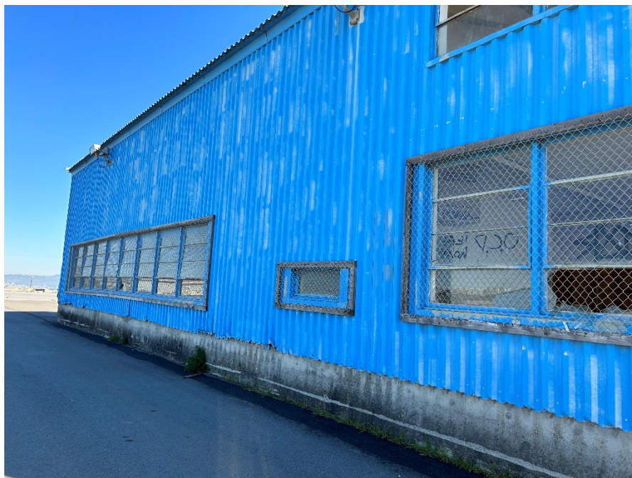
Parcel D-1 Photograph 10: Building 381, vegetation growth in the seam between exterior cover and building foundation. Facing northeast.
