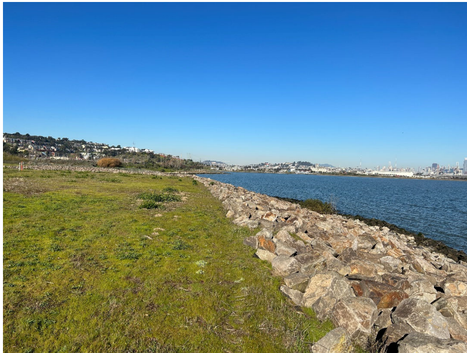
IR-07/18 Photograph 10: Shoreline revetment northwest of Building 146. Facing northwest. Photographed by: Marcella Navas/CH2M, 2/9/2023
