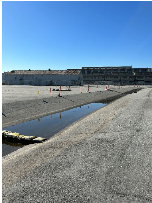
Parcel B-2 Photograph 4: Swale east of Building 130. Facing south. Photographed by: Marcella Navas/CH2M, 2/9/2023
