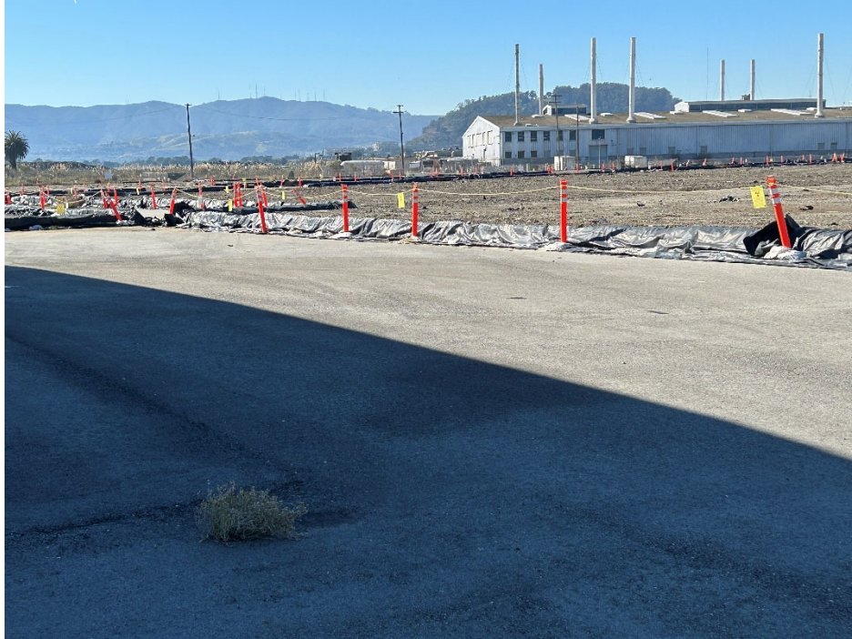
Parcel D-1 Photograph 11: Stormwater management best management practices southwest of Building 307. Facing southwest.
