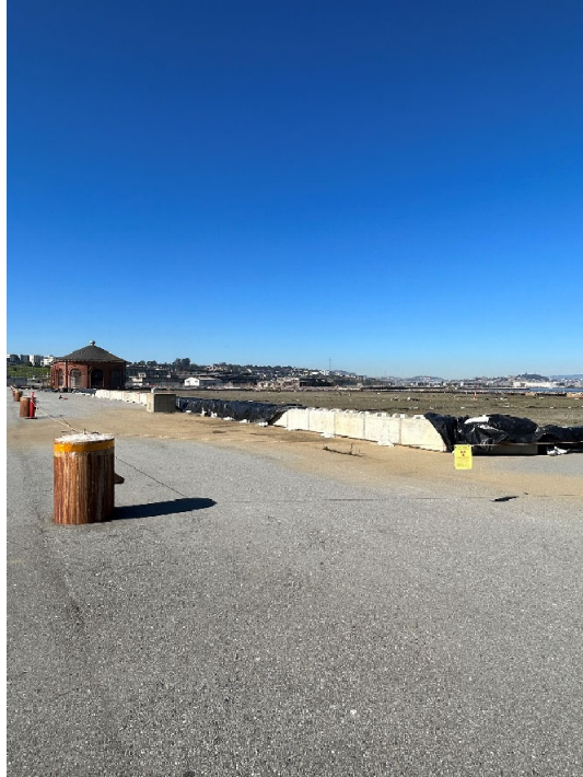
Parcel B-2 Photograph 15: Asphalt pavement cover. Facing northwest. Photographed by: Marcella Navas/CH2M, 2/9/2023
