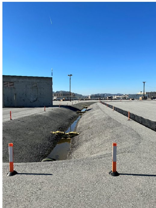
Parcel C Photograph 10: Paved drainage swale outfall south of Building 230. Facing southwest.
