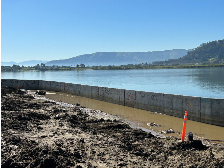
Parcel E-2 Photograph 9: Accumulated water behind seawall in active construction area. Facing southeast.
