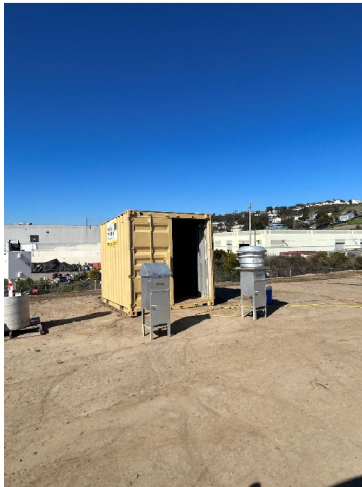
Parcel E-2 Photograph 2: Storage containers onsite for generators. Facing southwest. Photographed by: Marcella Navas/CH2M, 2/9/2023
