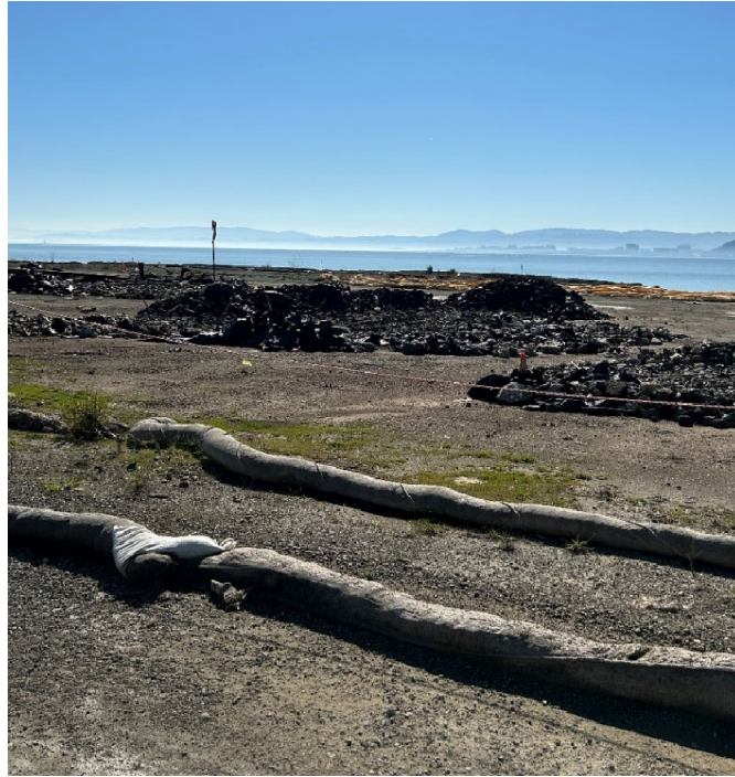
Parcel E Photograph 15: Stockpiles along embankment. Facing southeast. Photographed by: Marcella Navas/CH2M, 2/9/2023
