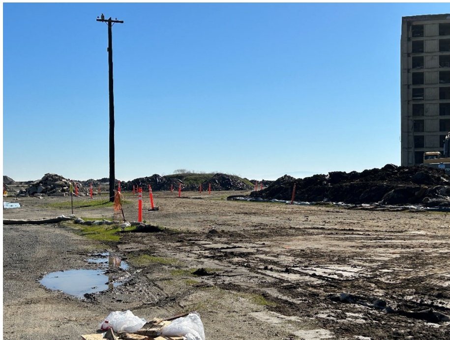
Parcel E Photograph 14: Overview of active construction area. Facing northeast. Photographed by: Marcella Navas/CH2M, 2/9/2023
