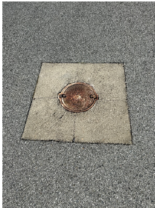
Parcel B-2 Photograph 12: Monitoring well. Facing southwest. Photographed by: Marcella Navas/CH2M, 2/9/2023
