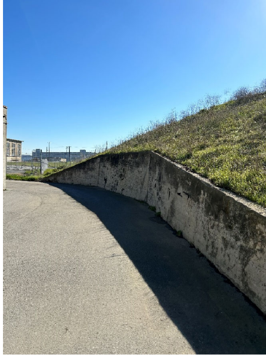
Parcel B-1 Photograph 1: Retaining wall southwest of Building 113. Facing southeast. Photographed by: Marcella Navas/CH2M, 2/9/2023
