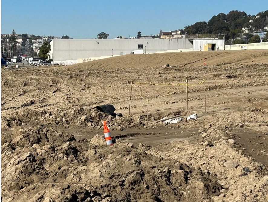
Parcel E-2 Photograph 3: Small excavated area within soil cover construction area. Facing southwest.
