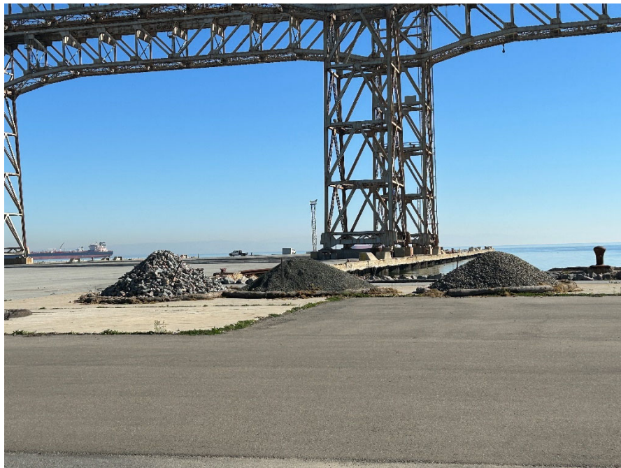
Parcel D-1 Photograph 20: Stockpiles from ongoing work with best management practices surrounding. Facing northeast.
