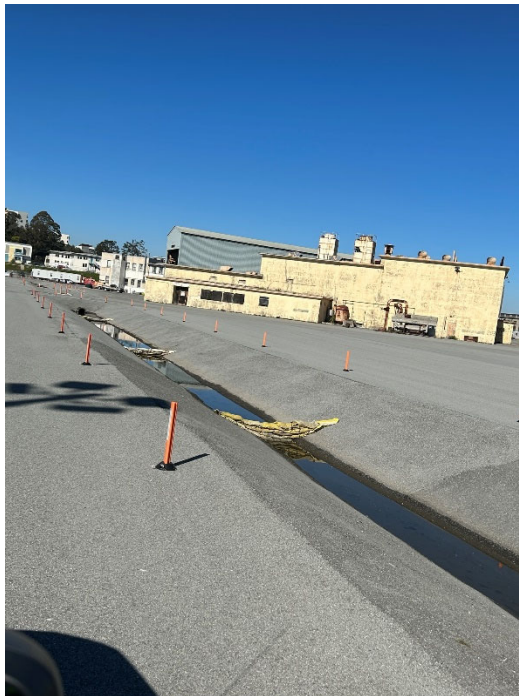
Parcel C Photograph 14: Paved drainage swale southeast of Building 235. Outfall south of Building 234. Facing northwest. Photographed by: Marcella Navas/CH2M, 2/9/2023
