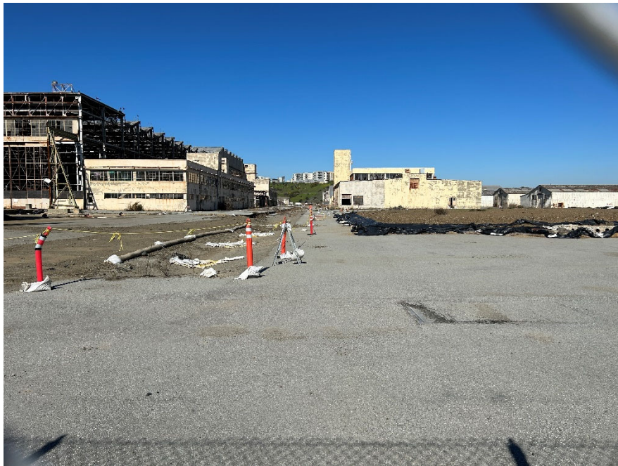
Parcel G Photograph 14: Asphalt pavement cover, trenching, and stormwater best management practices southeast of Building 411. Facing northwest. Photographed by: Marcella Navas/CH2M, 2/9/2023
