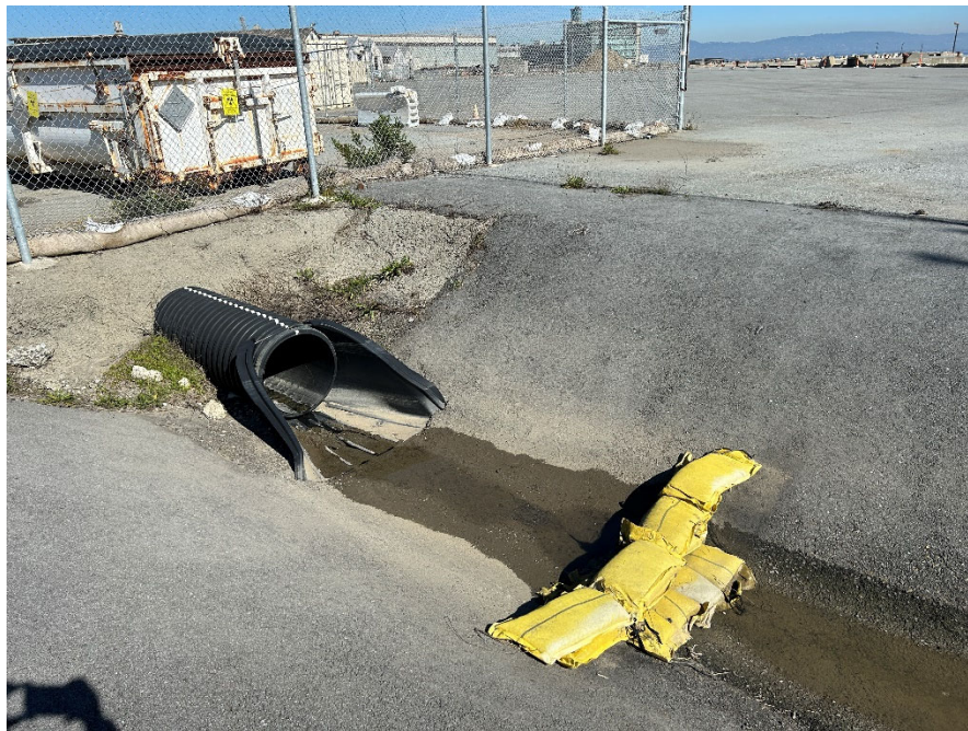
Parcel D-1 Photograph 8: Drainage swale adjacent to Parcel G. Minor vegetation growth in cracks along the seam between swale material and flat surface material. Facing northwest.
