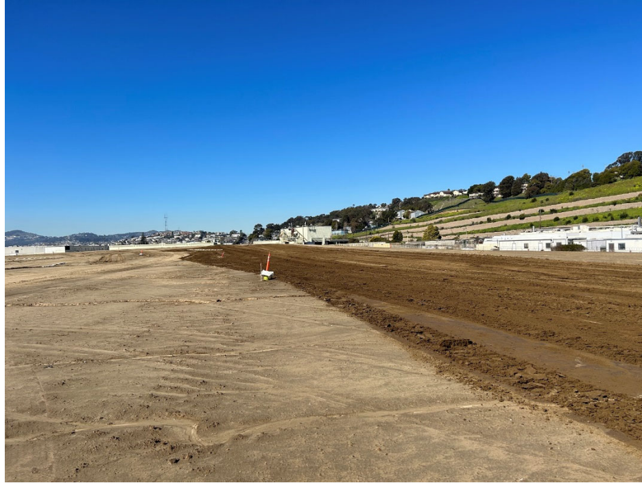
Parcel E-2 Photograph 5: Graded area with marked monitoring point. Facing southeast. Photographed by: Marcella Navas/CH2M, 2/9/2023
