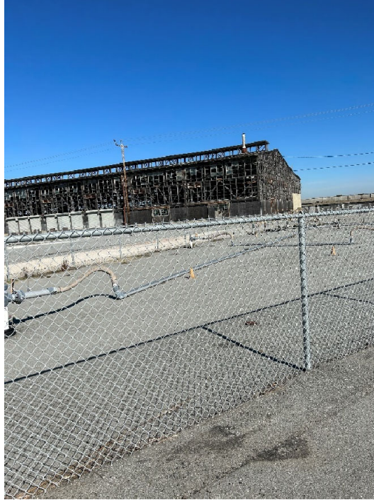
Parcel C Photograph 5: SVE treatment systems surrounded by chain-link fence. Facing northwest.
