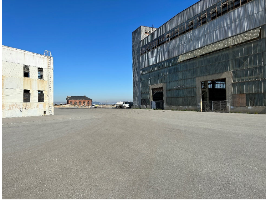
Parcel C Photograph 7: Asphalt pavement cover southwest of Building 214 along Lockwood Avenue. Facing northwest.
