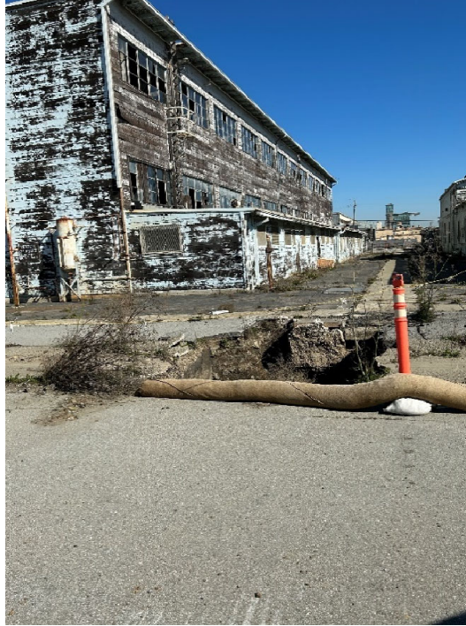
Parcel G Photograph 1: Excavation between Building 302 and 303. Facing northeast. Photographed by: Marcella Navas/CH2M, 2/9/2023
