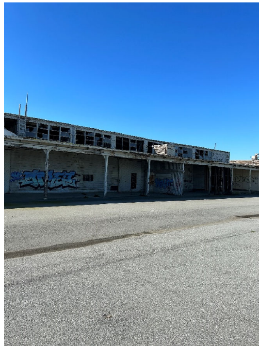
Parcel B-2 Photograph 2: Drainage swale in asphalt pavement cover and graffiti north of Building 128. Facing west.
