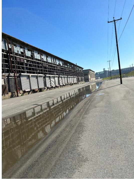
Parcel B-1 Photograph 7: Drainage swale in asphalt pavement cover southwest of Building 123, with accumulation of water. Facing southeast. Photographed by: Marcella Navas/CH2M, 2/9/2023
