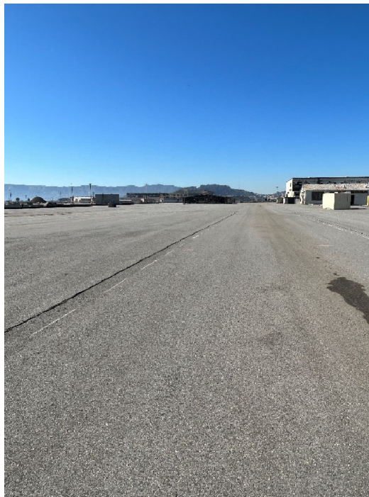
Parcel C Photograph 16: Asphalt pavement cover southeast of Building 228 along Nimitz Avenue. Facing southwest.
