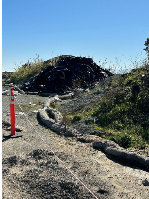
Parcel E Photograph 7: Stockpile near shoreline southeast of J Street. Facing southeast.
