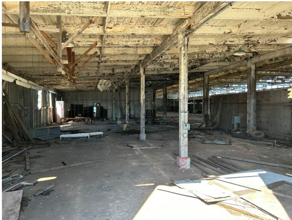
Parcel B-2 Photograph 10: View of the Building 128 foundation. Facing northwest. Photographed by: Marcella Navas/CH2M, 2/9/2023
