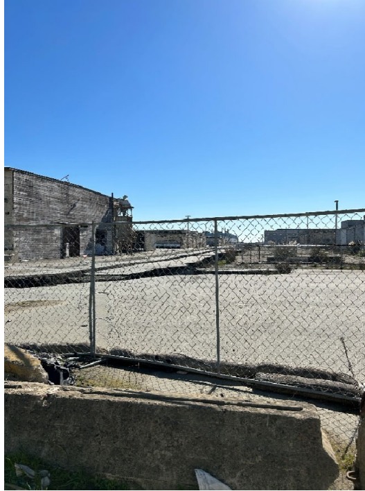
Parcel UC-1 Photograph 1: Chain-link fence along Parcel UC-1 and Parcel G. Facing south.
