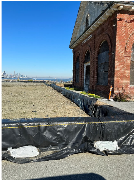
Parcel B-2 Photograph 14: Construction area with containment west of Building 140. Facing northeast. Photographed by: Marcella Navas/CH2M, 2/9/2023
