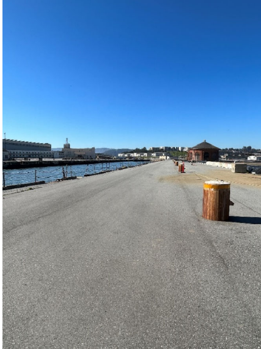
Parcel B-2 Photograph 13: Asphalt pavement cover. Facing west. Photographed by: Marcella Navas/CH2M, 2/9/2023
