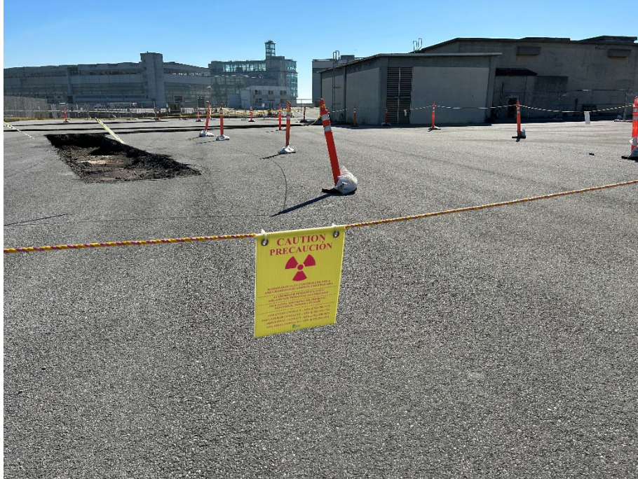
Parcel C Photograph 19: Signs signaling caution near trenching between of Building 134 and 135 outside of gated area of Parcel B-1. Facing southeast. Photographed by: Marcella Navas/CH2M, 2/9/2023
