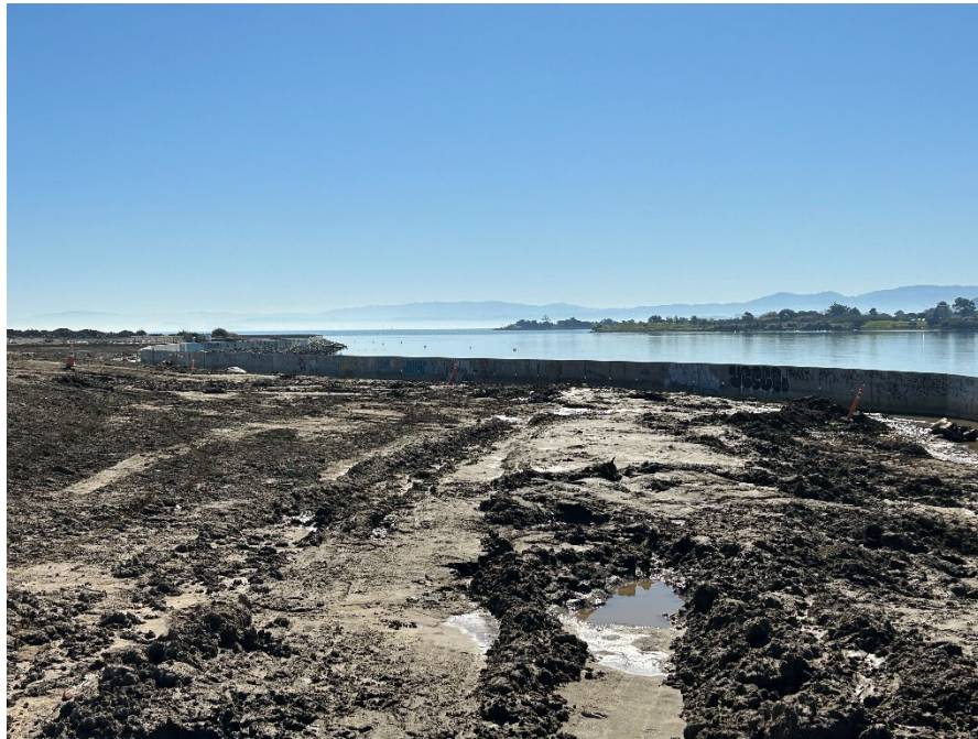
Parcel E-2 Photograph 12: Active soil cover construction area with seawall in the background. Facing southeast. Photographed by: Marcella Navas/CH2M, 2/9/2023
