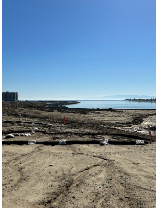
Parcel E-2 Photograph 1: Active construction with stormwater best management practices. Facing southeast. Photographed by: Marcella Navas/CH2M, 2/9/2023
