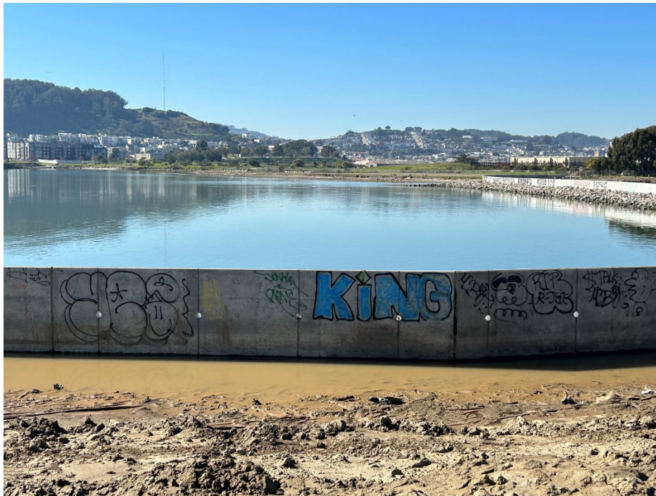
Parcel E-2 Photograph 10: Graffiti along seawall. Facing southwest.
