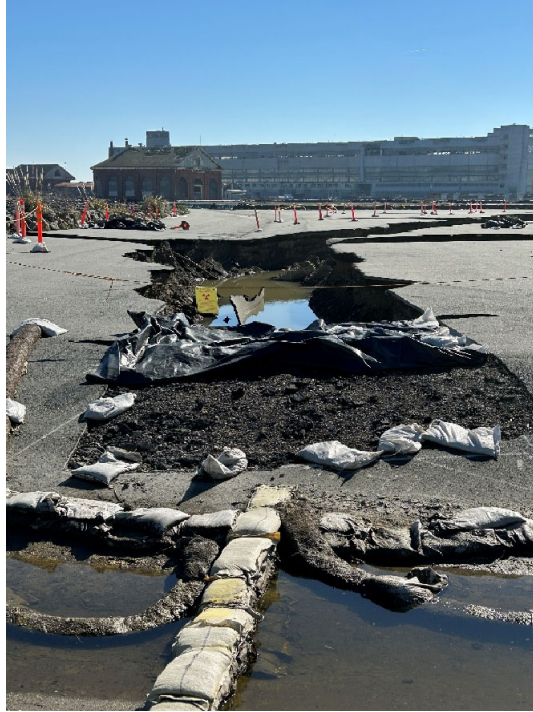
Parcel B-2 Photograph 5: Trenching east of Building 130 located south of outfall. Facing east.
