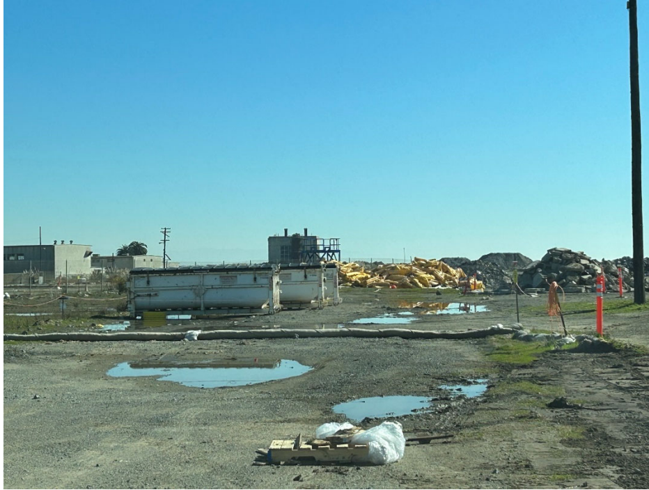
Parcel E-2 Photograph 15: Stockpiles along J Street with swale surrounding. Facing northeast.
