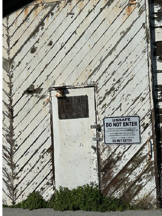
Parcel B-2 Photograph 9: Do Not Enter sign and locked door, Building 128. Facing north Photographed by: Marcella Navas/CH2M, 2/9/2023
