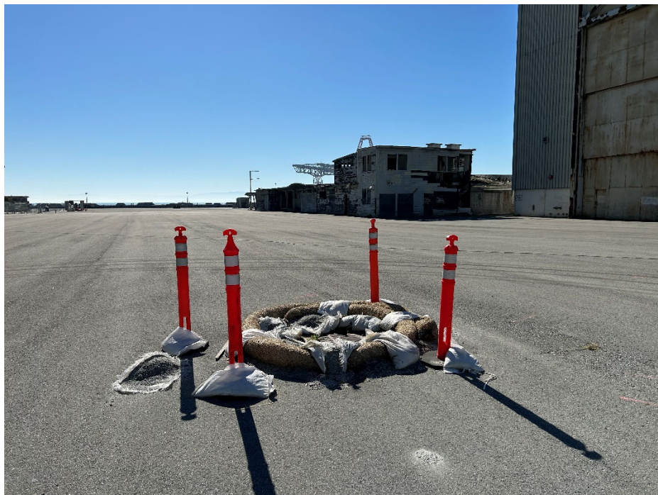
Parcel C Photograph 12: Stormwater best management practice around catch basin west of Building 231. Facing southeast.
