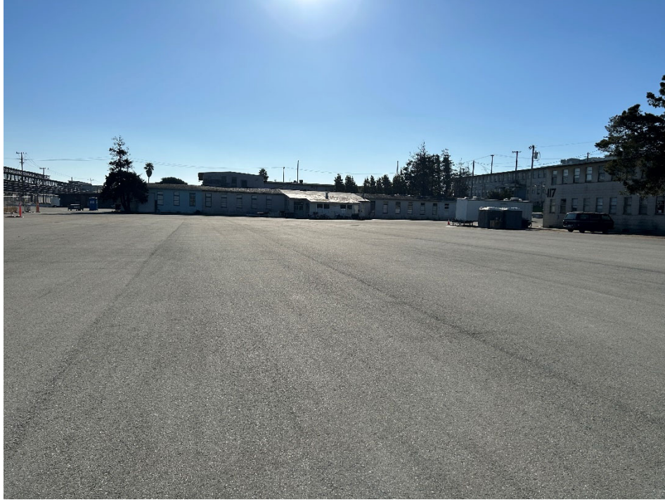
Parcel B-1 Photograph 5: Asphalt pavement cover southwest of Building 121. Cover is generally intact and in good condition. Facing east.
