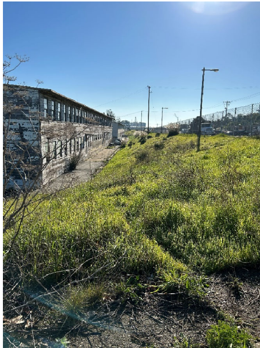
Parcel B-1 Photograph 2: Soil cover southwest of Building 103 adjacent to Galvez Avenue. Facing southeast. Photographed by: Marcella Navas/CH2M, 2/9/2023
