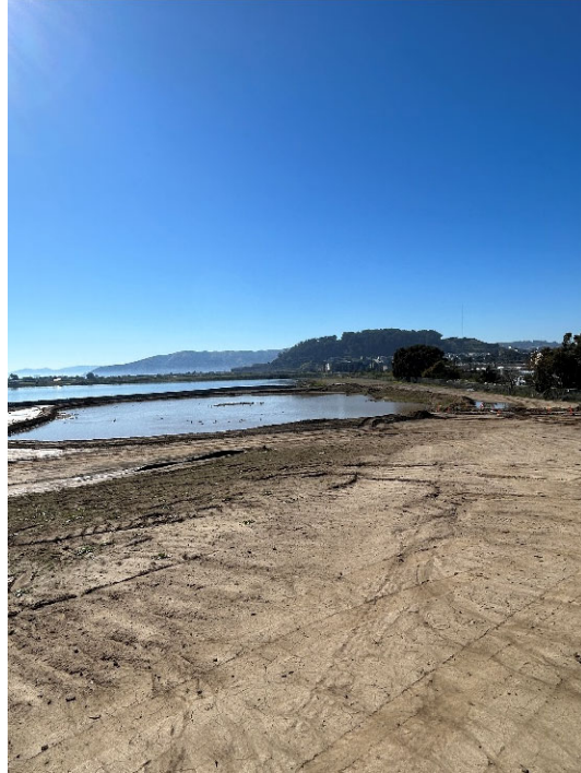
Parcel E-2 Photograph 13: Accumulated water within retention area, active construction site. Facing southwest.
