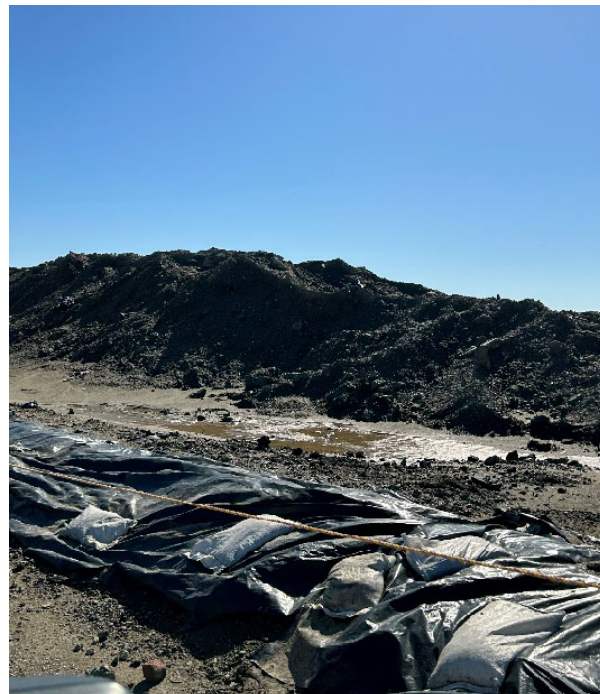
Parcel E-2 Photograph 14: Stockpile along J Street surrounded by stormwater best management practices. Facing southeast.
