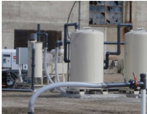
An extraction system removed vapors from the soil
