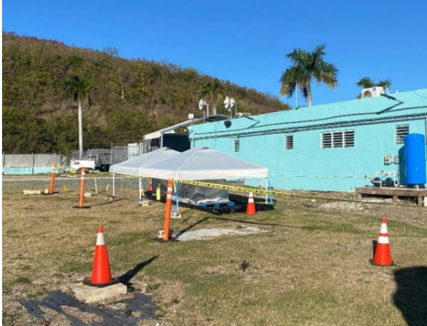
Sunshade over EVO containers
