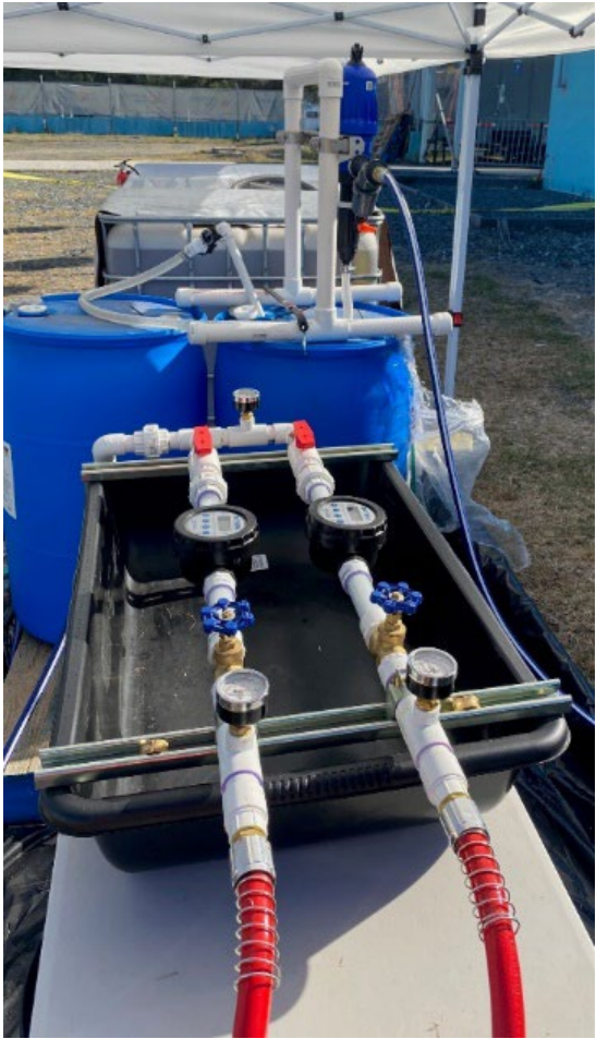
Injection Manifold and Dosatron
