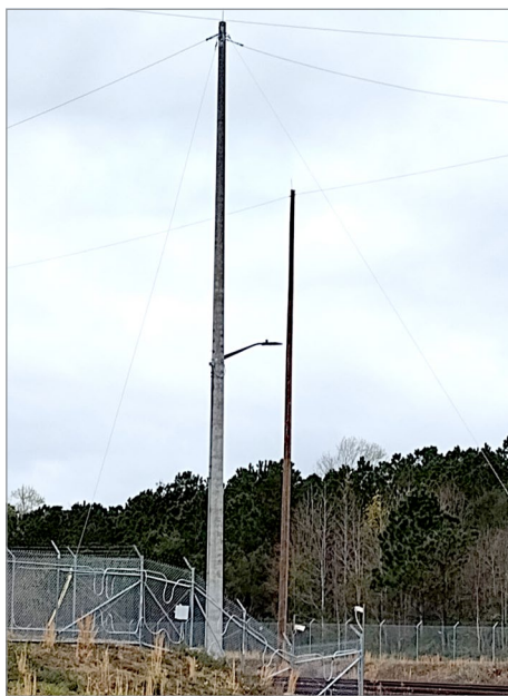
Figure 3. Concrete (left) and Wooden (right) Poles at MOTSU Source: The DoD OIG.
