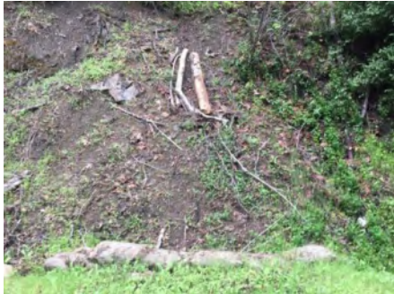
Photo 1. Culvert inlet. Note landslide above inlet. (March 2021).
