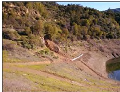
Photo 4. Gullying on Austrian Dam (Feb. 2016)
