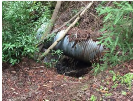
Photo 2. Culvert outlet. Note erosion (March 2021).
