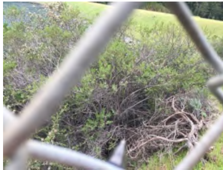
Photo 2. Culvert outlet shown by pencil ( March 2021 ).
