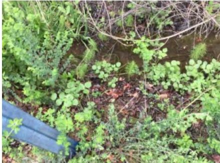
Photo 1. Buried/damaged culvert inlet suspected below blue marker ( March 2021 ).
