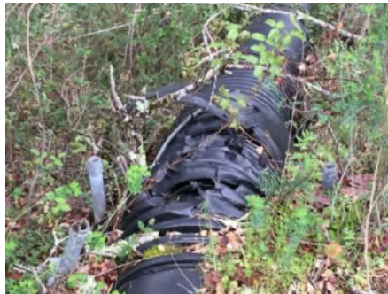
Photo 2. Culvert outlet in need of repair ( March 2021 ).
