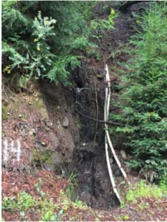
Photo 1. Erosion apparent at culvert inlet area (March 2021).
