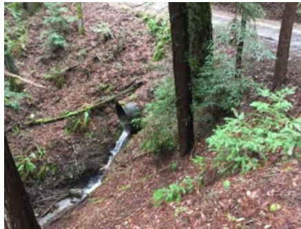
Photo 2. Culvert outlet area. Note erosion. ( March 2021 ).
