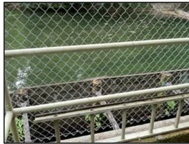
Photo 20. Wooden boards that protect the intake manifold at Ostwald Intake are rotting and in need of repair and replacement (Oct. 2013).
