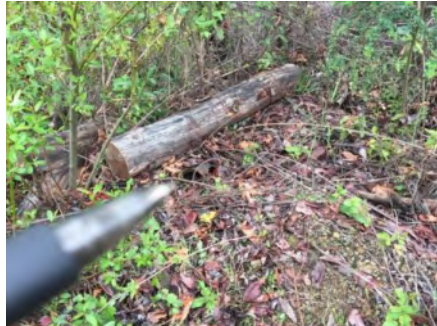
Photo 2. Suspected culvert outlet area. Pencil points to damaged piece of pipe ( March 2021 ).
