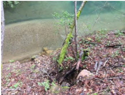
Photo 2. Culvert outlet and erosion ( March 2021 ).
