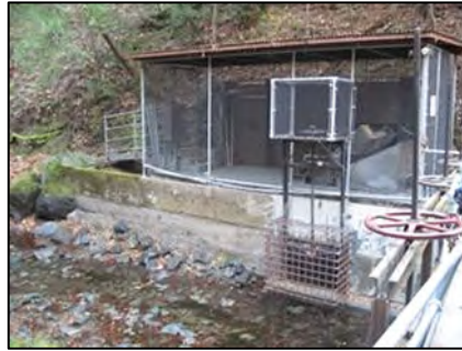
Photo 37. Intake gate and leaf screening facility at Lower Cavaneer Intake Facility (Dec. 2013).
