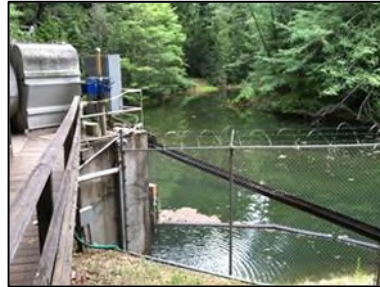
Photo 19. Inflated rubber dam on Los Gatos Creek provides an adequate pool elevation for the Ostwald Intake (Oct. 2013).
