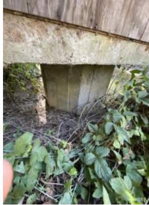
Photo 50. Aldercroft Heights Extraction Well pump pillar (Aug. 2021).
