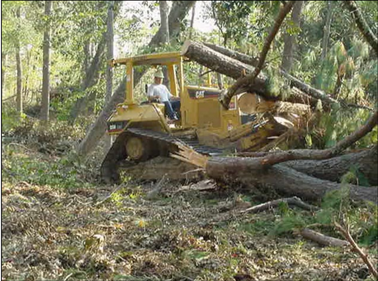
Photo 6.1 Post Hurricane Rita debris cleanup.
