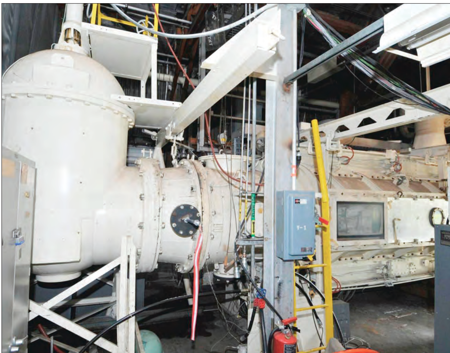
The main tunnel control valve of the 1-foot transonic wind tunnel, 1T, at Arnold Air Force Base, is pictured here to the left, and from there the air flows to the test section. In October 1952, 1T was the first operational wind tunnel at Arnold. (U.S. Air Force photo)
