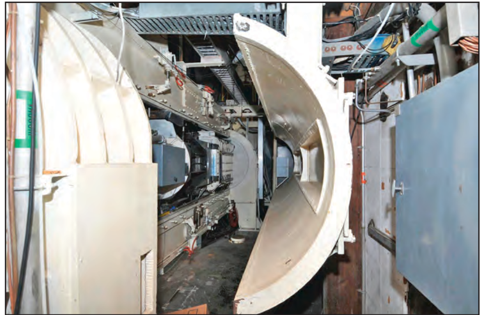
With the plenum shell retracted, the inside of the test section is visible in the 1-foot transonic wind tunnel, or 1T, at Arnold Air Force Base. The wind tunnel still exists but is no longer operational. From 1952 until its last test in 1995, approximately 400 tests were conducted. (U.S. Air Force photo)
