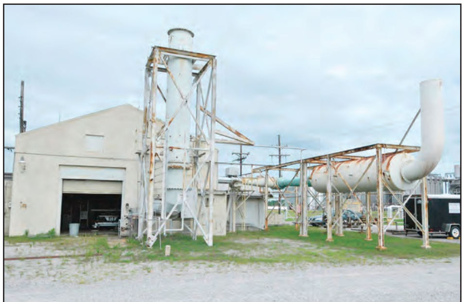
The structure to the left is the main flow exhaust for the 1-foot transonic wind tunnel at Arnold Air Force Base, and at right is the steam ejector exhaust for the tunnel. 1T was operational beginning in October 1952. Its last test was conducted in 1995. (U.S. Air Force photo)
