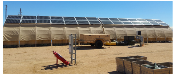
Lackland AFB, Texas. At expeditionary microgrid system at Lackland AFB, monocrystalline silicon solar panels are placed on top of each tent for energy production while a trailer (center) holds the hardware, software, and lithium-ion batteries that form the smart grid. U.S. Air Force Photo by Donna Lindner. February 2, 2016.
