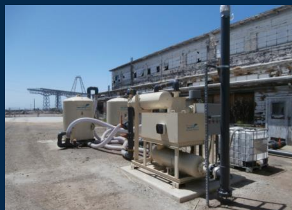
Soil Vapor Extraction at Parcel C
