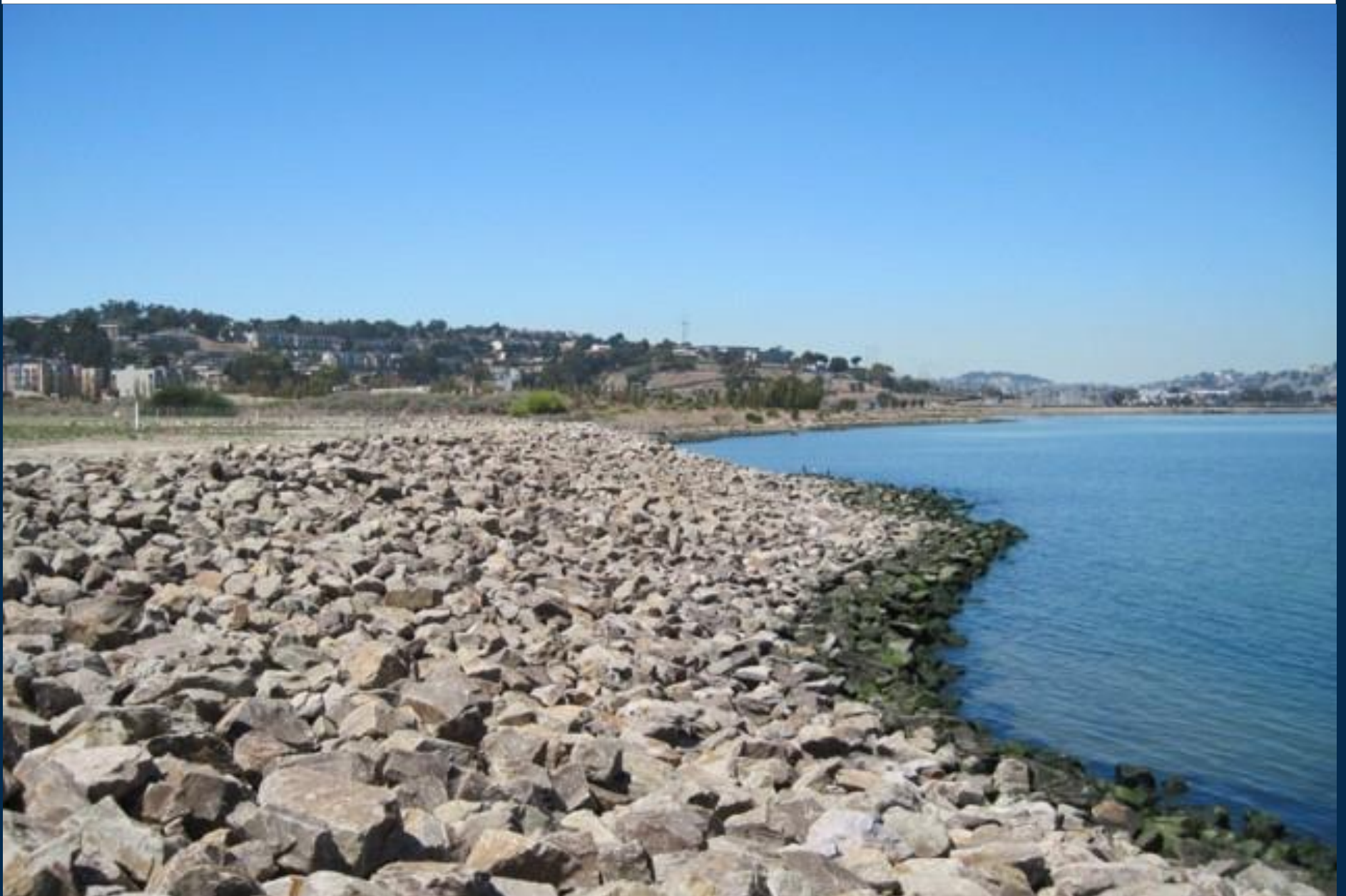
The remedy at Parcel B includes a rock barrier (known as a revetment ) to protect against shoreline erosion View from Parcel F finger piers off of Parcel B, looking towards new development on former Parcel A and neighboring private property
