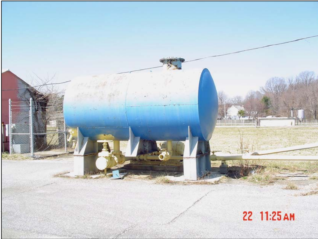
Photo 5: Aboveground Water Storage tank on property, which is empty and disconnected.
