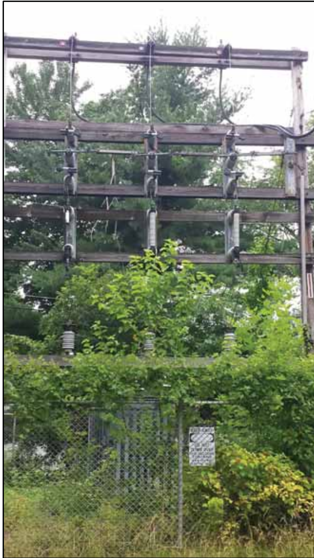
Photo 7 Power Transfer Station
