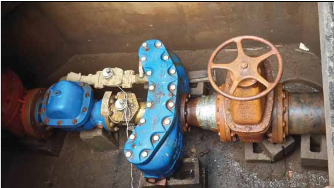
Photo 8 Water Main Valve
