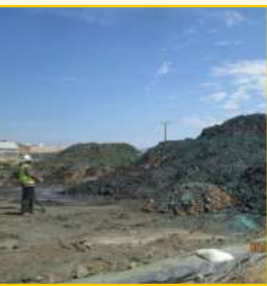
Stockpiles of soil are sprayed with a soil cementing compound to prevent windblown dust
