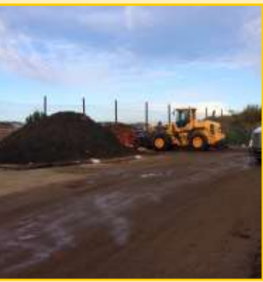
Straw waddles are placed at the base of soil stockpiles to prevent runoff during heavy rains
