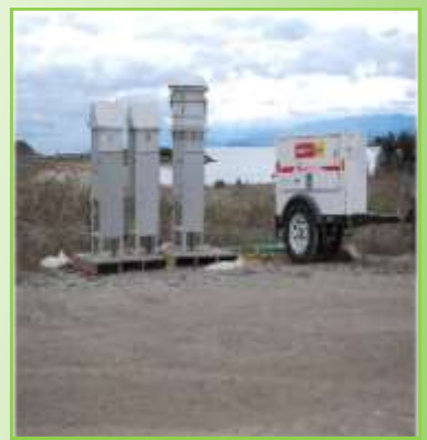
Air monitoring equipment is placed in work areas with ongoing construction activities
