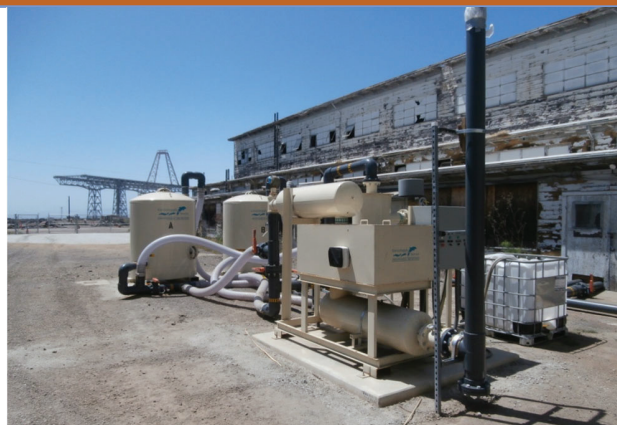
Soil vapor extraction (SVE) at Parcel C
