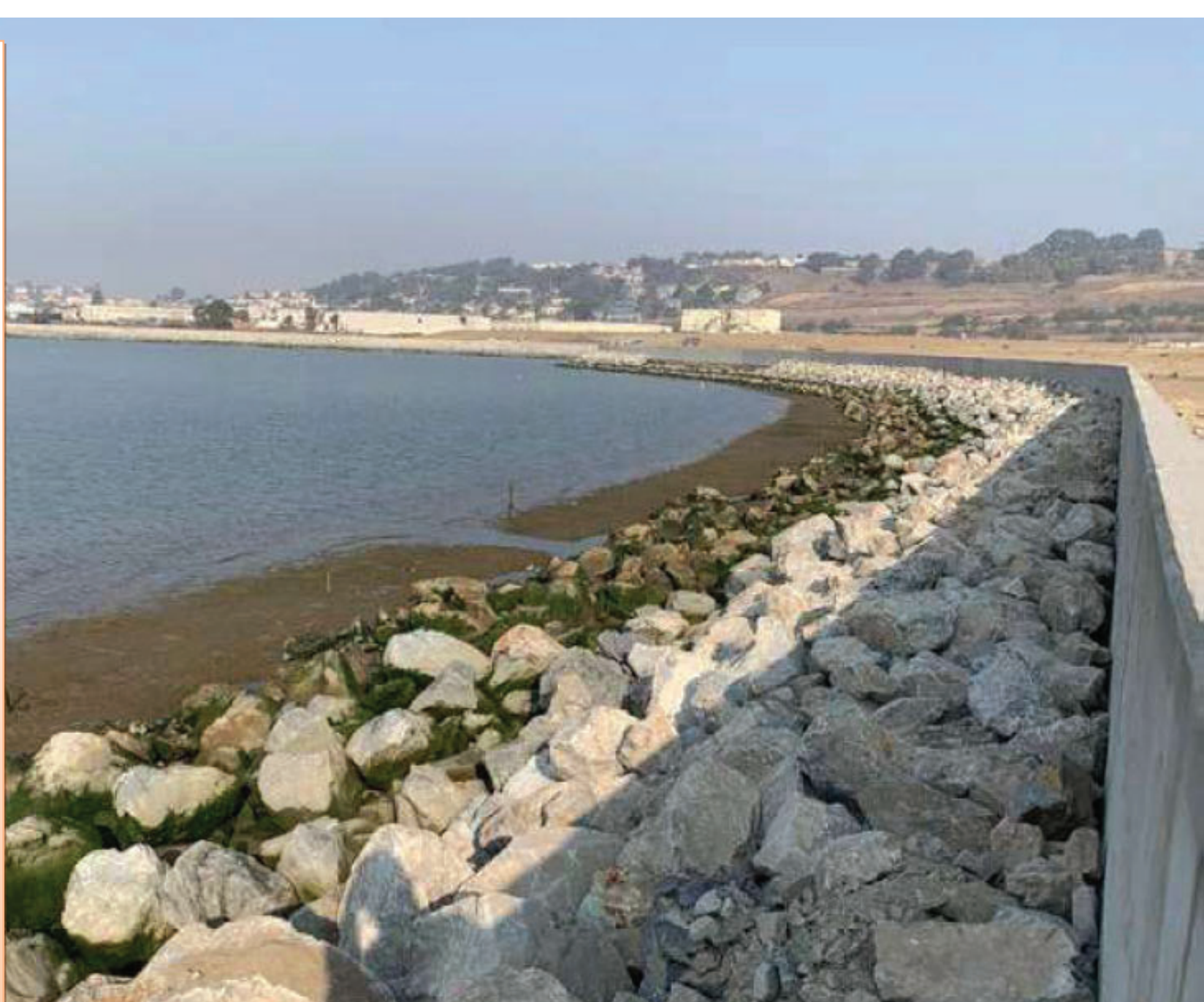
View of final revetment and sea wall at Parcel E-2 (looking northwest)
