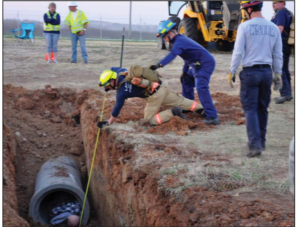
A search and rescue team works to recover simulated victims from a collapsed trench, one of the newest training venues at Crisis City. (Photo by Sgt. 1st Class Jeremy Byers, Public Affairs Office)
