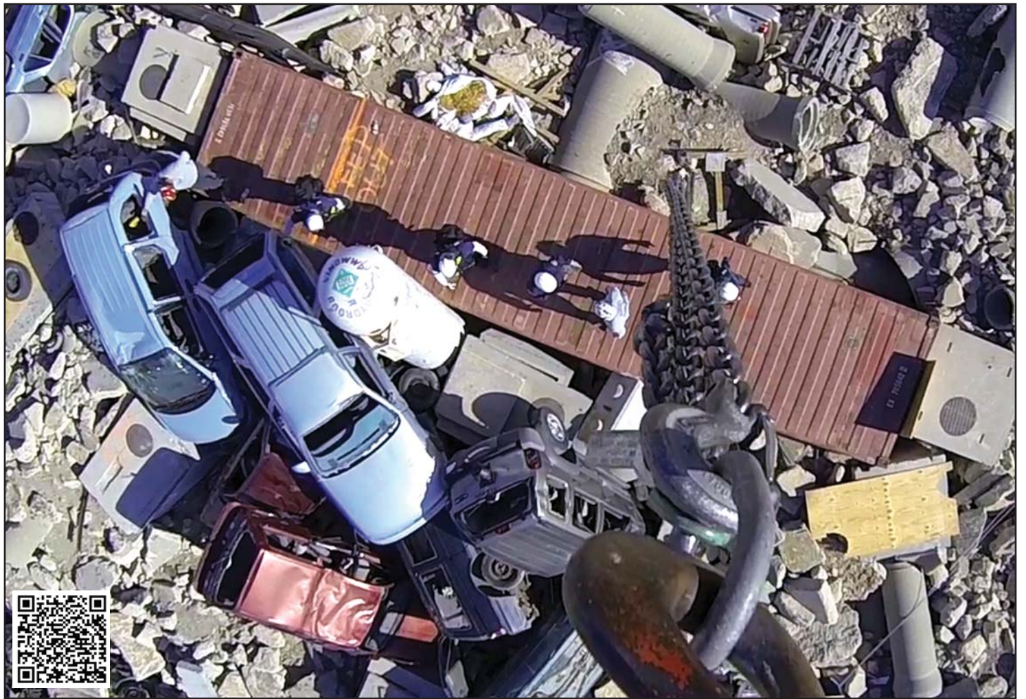
A crane’s-eye view of rescue operations illustrates the realistic nature of the obstacles facing search and rescue workers on the collapsed building venue at Crisis City March 31-April 1 during a full-scale exercise. First responders from across the state took part in the two-day exercise. (Photo by Sgt. Zach Sheely, Public Affairs Office)
