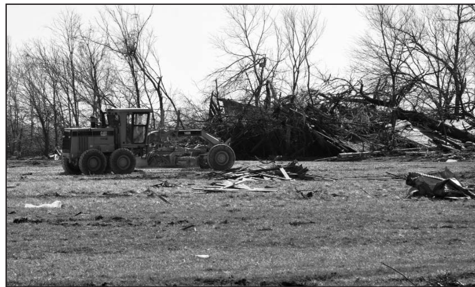
Debris generated by the 2012 Harveyville tornado is collected and deposited in a designated dump site on the outskirts of the town. (Photo by 1st Lt. Matt Lucht, Public Affairs Office)
