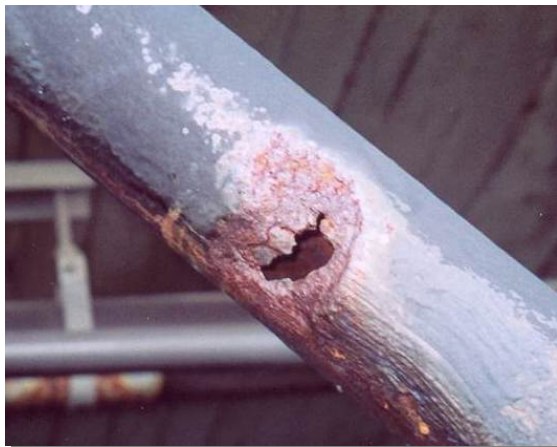
Photo 3-2 - Diagonal Bracing, Corrosion Hole
