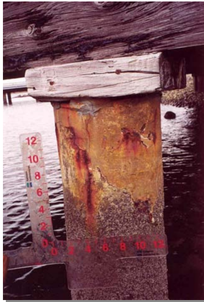
Photo 4-1 - Rust Staining of Concrete Pile
