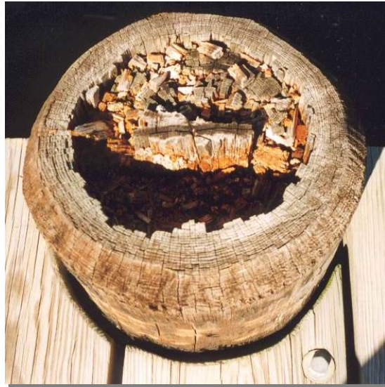
Photo 2-1 - Fungal Rot of a Timber Pile
