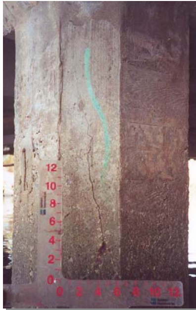
Photo 4-3 - Vertical Cracking in Tide Zone
