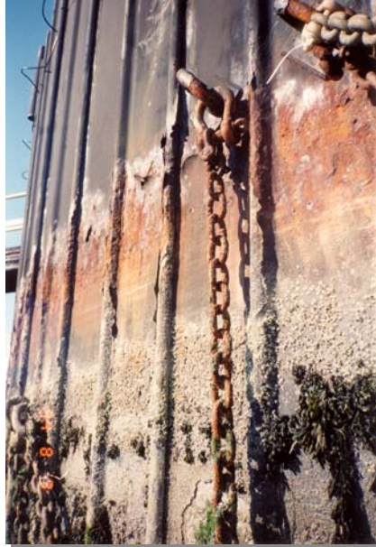
Photo 3-7 - Coating Deterioration in the Splash Zone
