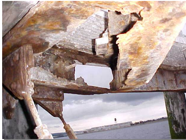
Photo 3-4 - Severely Corroded Steel Framing
