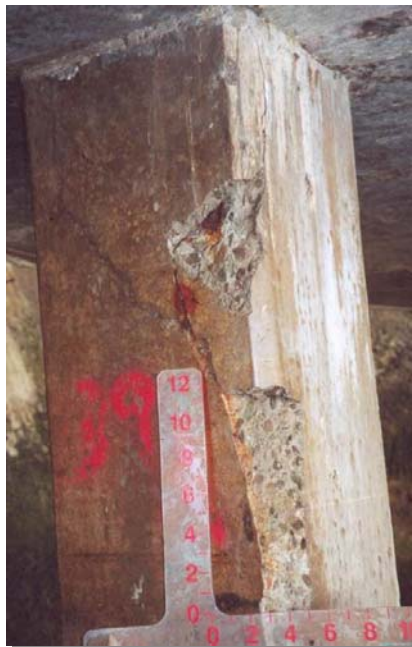
Photo 4-2 - Vertical Crack and Spall
