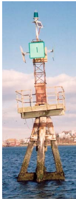
Photo 2-4 - Structure Alignment Problem
