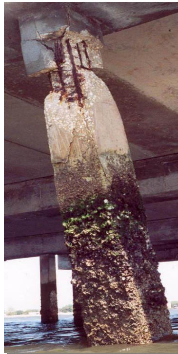
Photo 4-4 - Failed Repair with Exposed and Corroded Reinforcing
