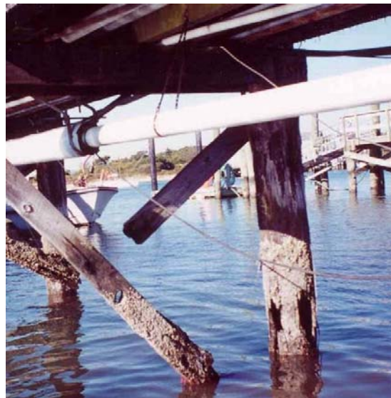
Photo 2-2 - Marine Borer Deterioration of Bracing and Pile in the Tidal Zone
