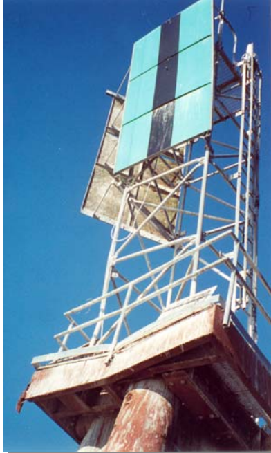
Photo 3-5 - Vessel Impact Damage to a Fixed ATON Structure
