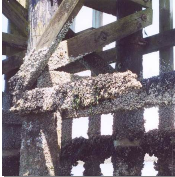
Photo 2-3 - Deterioration of Longitudinal Wale
