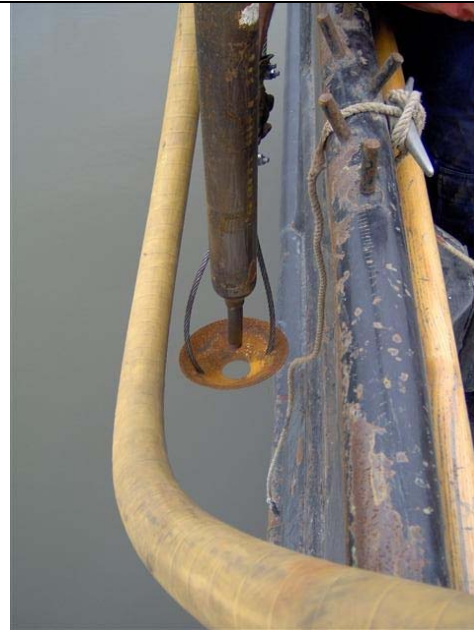
Figure 11-6 Jet Pipe Over the Side
