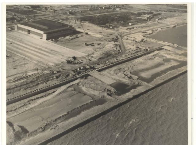
Hangar 41 nears completion, while the waterfront area is dammed to construct the ramps, 1941. (NAS Corpus Christi, Public Affairs Office)
