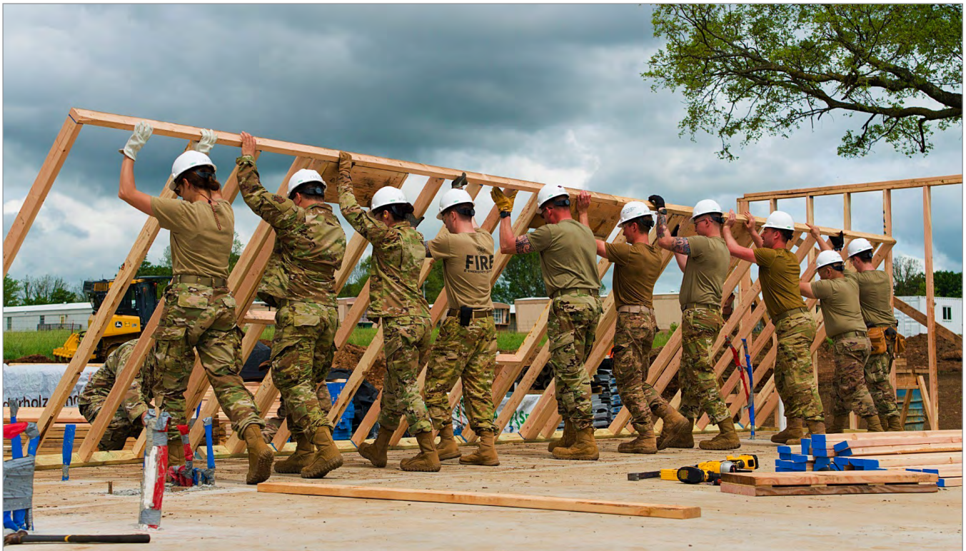
Airmen construct the first home in the Cherokee Veterans Housing Initiative in Tahlequah, Oklahoma, on May 18, 2021.
