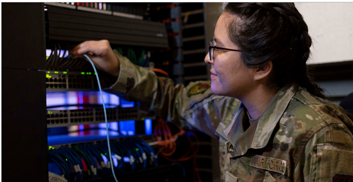
An Airman with the 60th Communications Squadron configures a switch at Travis Air Force Base, California, on September 23, 2021. Source: The Air Force.
