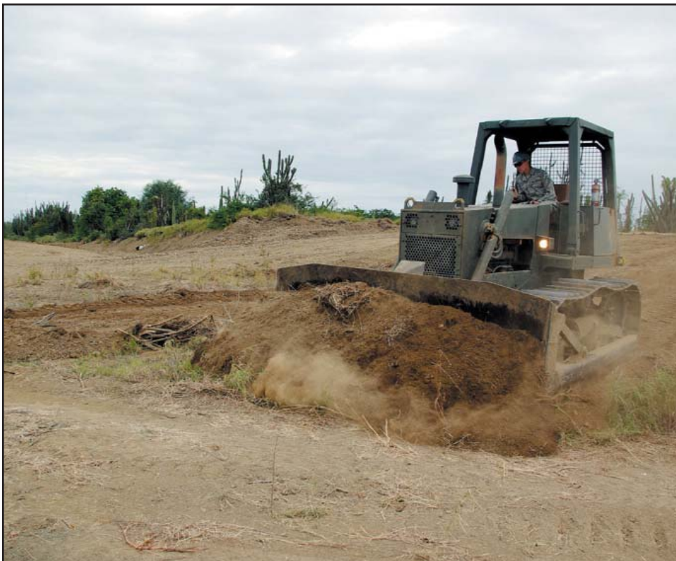
An Airman from the 190th Civil Engineering Squadron, Kansas National Guard, used a bulldozer to clear land near Guantanamo Bay, Cuba, to prepare the area for Haitian relief operations. (Photo by Senior Airman John Countryman)
