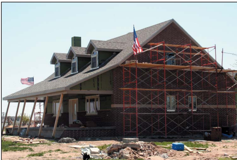
Every house that goes up in Greensburg is another sign that the town, once nearly destroyed, is on the road to recovery. (Photo by Sharon Watson)
