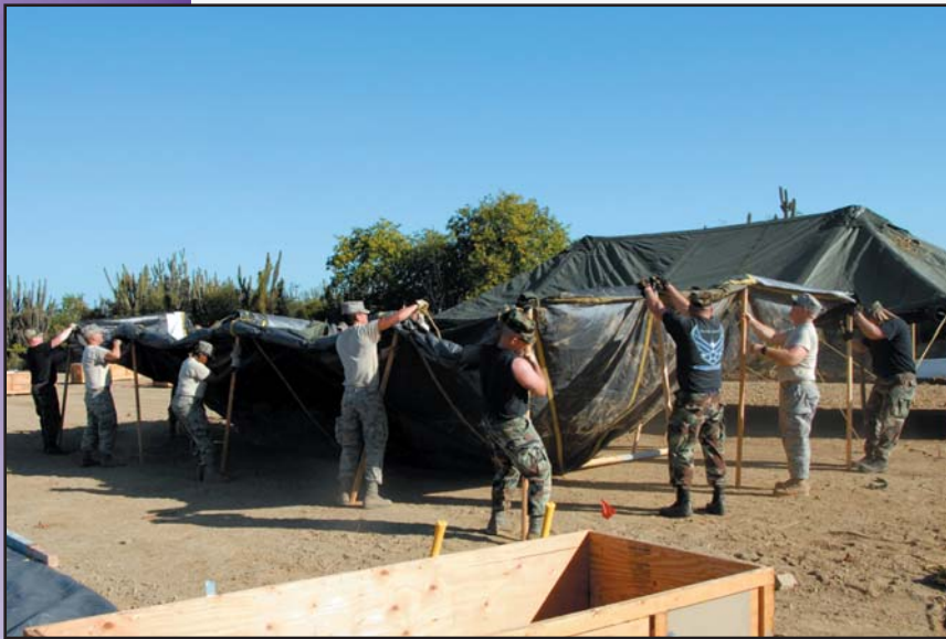
Members of the 190th Civil Engineering Squadron assemble a tent in Cuba for refugees from the Haitian earthquake in January 2010.
