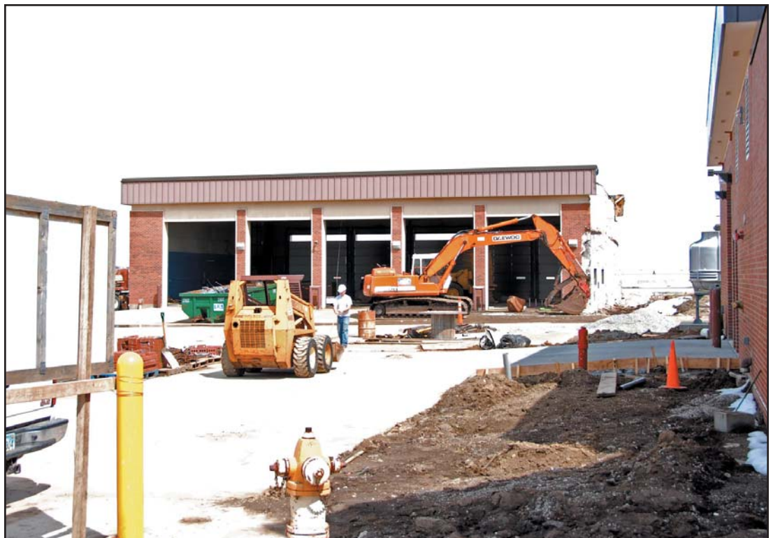
A new fire station is under construction at the 190th Air Refueling Wing in Topeka. The new facility will enhance the wing’s ability to respond to fires on base.
