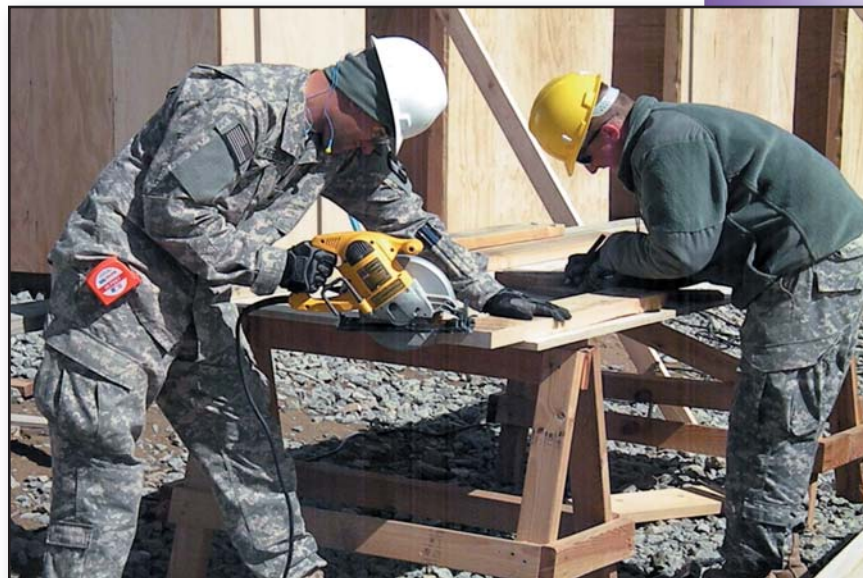
Sgt. Matthew Pierson and Spc. Kyler Wellman work on measuring and cutting structural pieces needed to build a 16-room Super B hut for their detachment at Forward Operating Base Sharana, Afghanistan.
