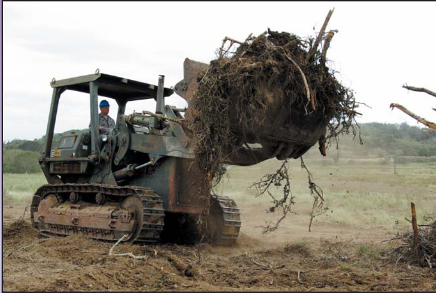
Members of the 190th Air Refueling Wing Civil Engineering Squadron were tasked with preparing the ground and constructing temporary housing at Guantanamo Bay, Cuba, for Haitian refugees following the earthquake that struck Haiti in January 2010.
