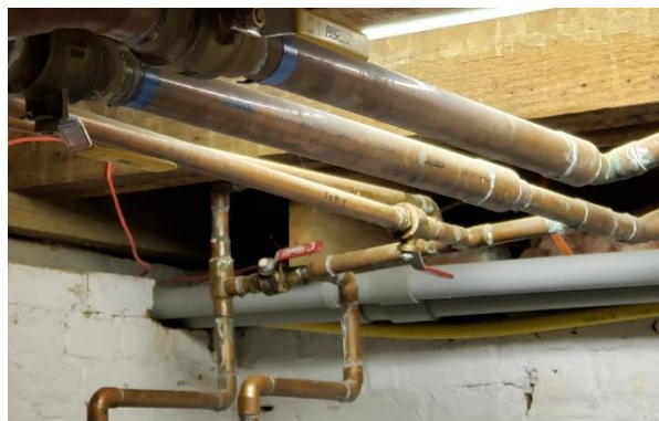
Image showing residential copper water lines and fittings
