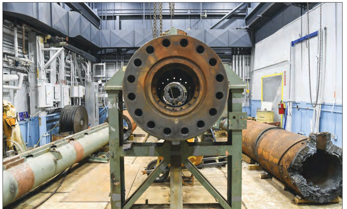
Prior to their removal, disassembled pieces of Tunnel E sit in a building that housed the old wind tunnel at the von Kármán Gas Dynamics Facility on Arnold Air Force Base, March 4. (U.S. Air Force photos by Jill Pickett)
