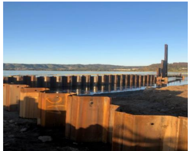
A sheet pile wall is the first step in ways the Navy will protect the shoreline at IR-03.
