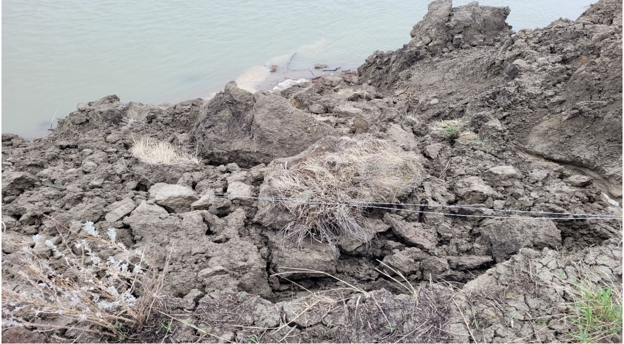
This barbwire fence was put up in the summer of 2020 around the slumping but is now part of the slumping.
