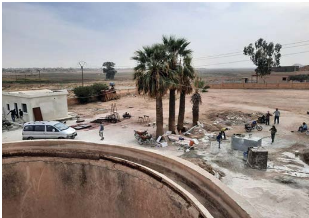
Rehabilitation of Shaddadi Desalination Plant will provide a sustainable water supply to an estimated 9,000 beneficiaries in al-Shaddadi. (USAID photo)
