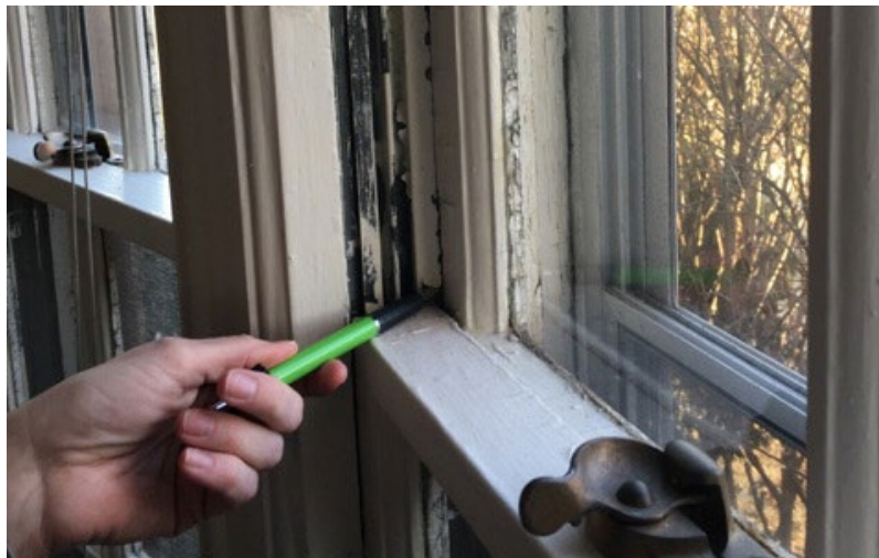
Figure 2. Presumed Lead-Based Paint Flaking on Window at Wright-Patterson AFB
