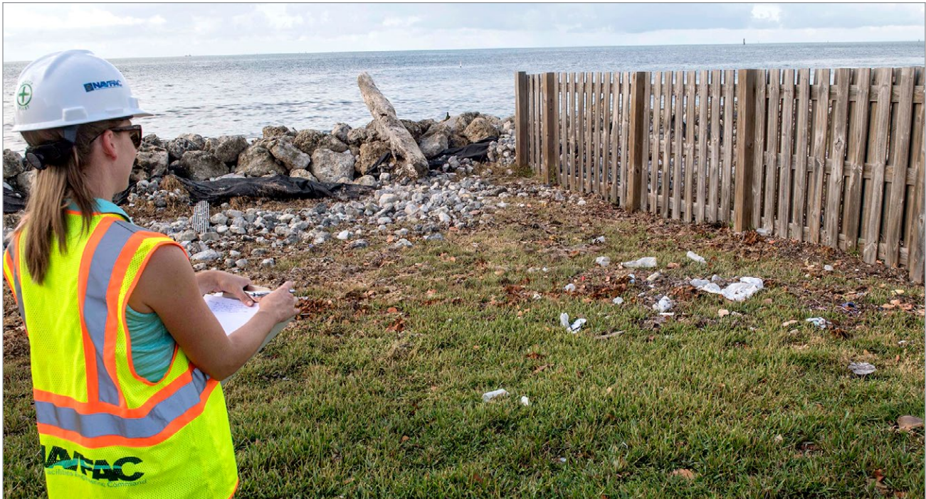
A structural engineer assigned to Naval Facilities Engineering Command (NAVFAC) Southeast records the damage to a fence on Naval Air Station Key West in the aftermath of Hurricane Irma Source: U.S. Navy.
