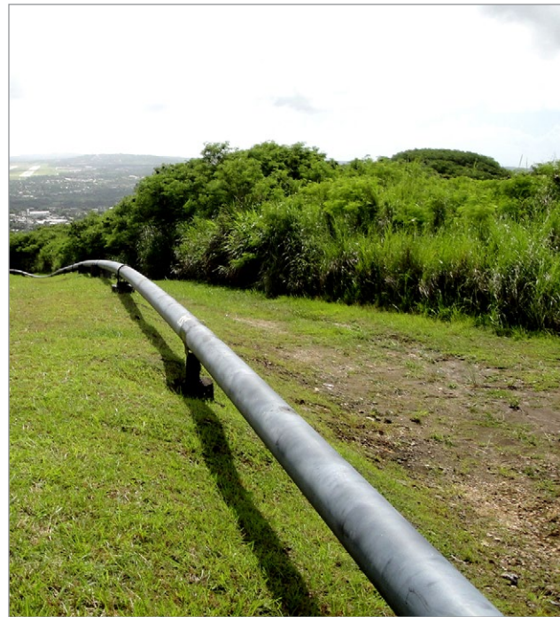
Fuel Pipeline on Guam Source: NAVFAC Marianas.
