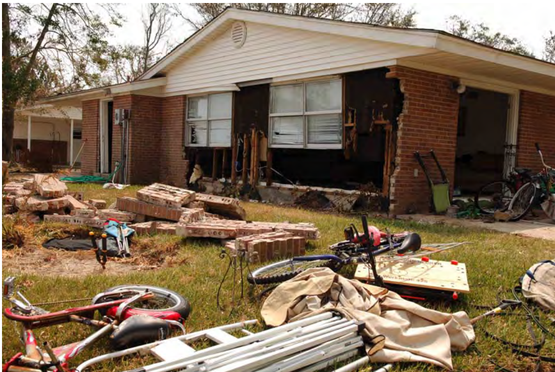
Personal belongings and parts of walls are strewn about the backyard of a home on the perimeter of the Bay Ridge housing area on Keesler AFB, Mississippi. Hurricane Katrina's high winds and storm surge downed trees, engulfed homes in debris and destroyed houses in the area (USAF photo by Joe Piccorossi).
