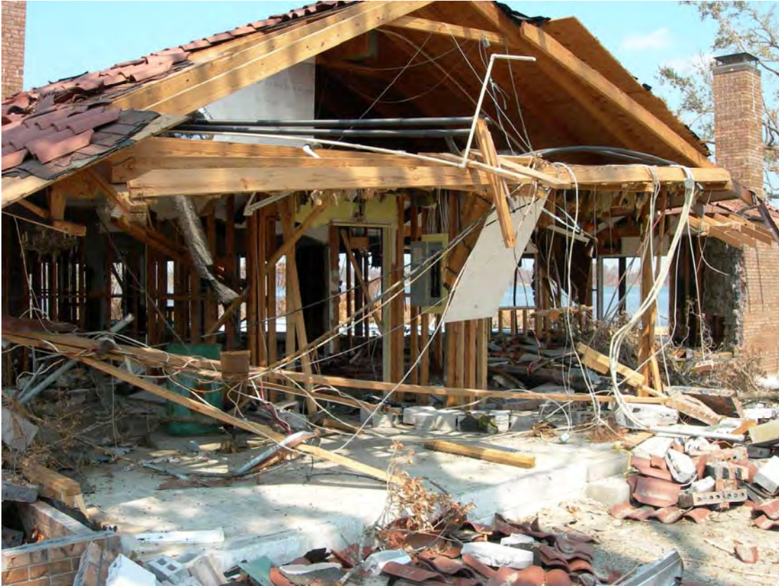
Military Family Housing units along the Back Bay of Biloxi were particularly hard hit by Hurricane Katrina's storm surge, which raised water levels nearly 20 feet, flooding approximately half of Keesler AFB, Mississippi. The sites with the lowest elevations above sea level were abandoned as Keesler planned to rebuild its housing units (photo by Capt Brady Smith).
