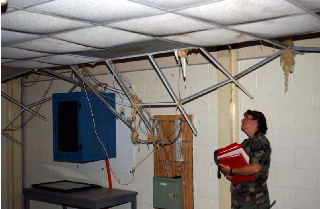
1st Lt Wendy Hendley, 403rd Wing facility manager, inspects damage for Air Force Reserve Command civil engineers during AFRC's assessment team visit to Keesler AFB, Mississippi, on 20 September 2005. Many of the command's office buildings, maintenance shops and hangars were severely damaged by Hurricane Katrina (USAF photo by Lt Col Bob Thompson).
