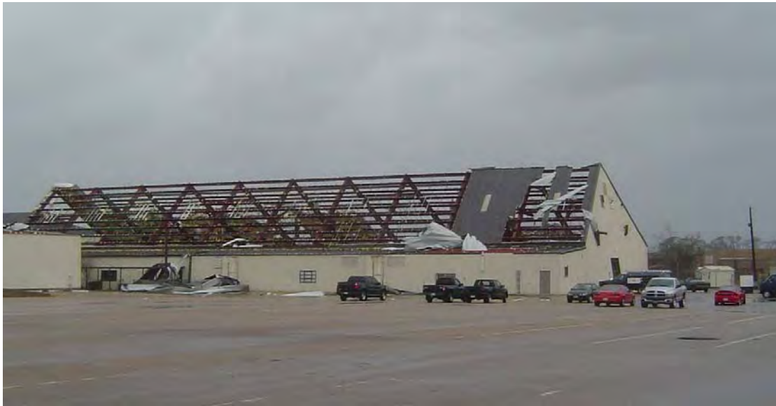
Winds gusting to 140 mph heavily damaged the older roofs on Keesler AFB. Newer construction fared better, because the more recent buildings had been designed to withstand Category 5 winds.
