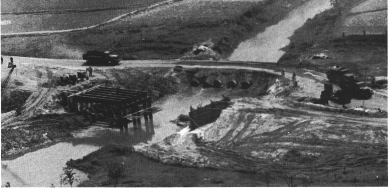
BRIDGING OVER —Aerial view shows one of the steel bridges being built by MCB-10 in the northern I Corps area.
