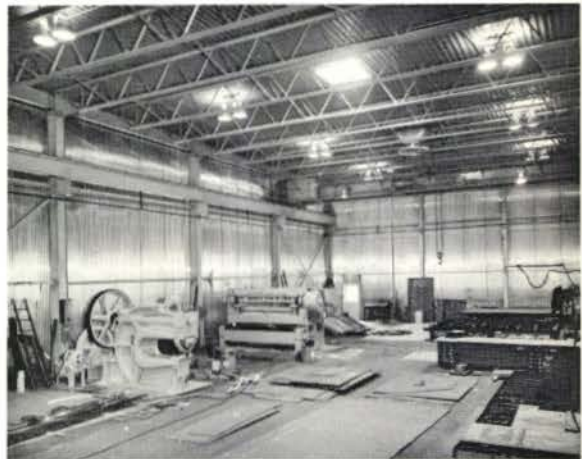
An example of mercury lighting in an industrial shop. Note good distribution of illumination. Photographs courtesy of the Holophane Company.
