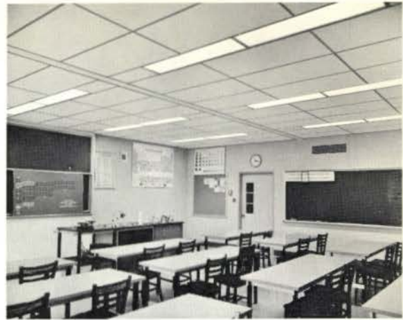
An example of good fluorescent lighting in a classroom. Troffer units are installed in a hung ceiling for better reflection and attractive appearance.
