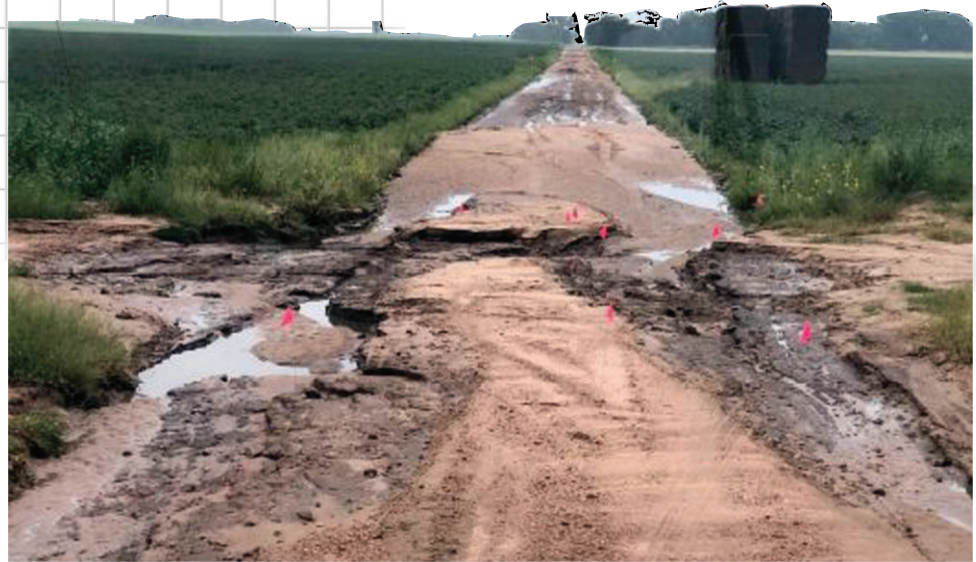
Heavy rains in September resulted in flooding in several counties, washing out roads and damaging bridges and other infrastructure.
