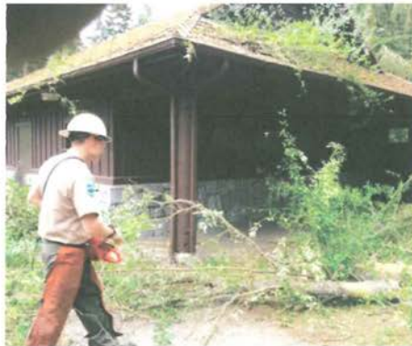
Ranger Ben Shook prepares to remove a tree from the roof of a restroom in the campground.
