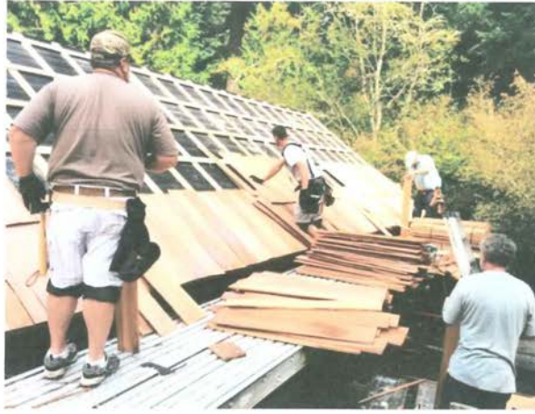
Dale, Craig, Joe, and Matt lay out shakes and nail them to the roof of the historic structure
