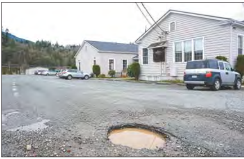
Potholes mar Lyman Avenue outside Lyman Elementary School. The town of Lyman has received a grant to repair the road.
