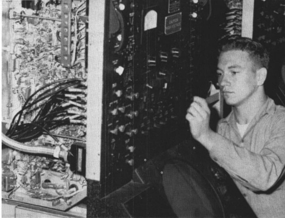
ELECTRICAL HAZARDS —Only qualified men should work on electrical gear.
