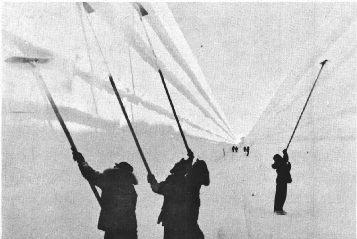
INSIDE JOB —Navymen scrape the loose snow from walls of main tunnel while building new base in Antarctica.
