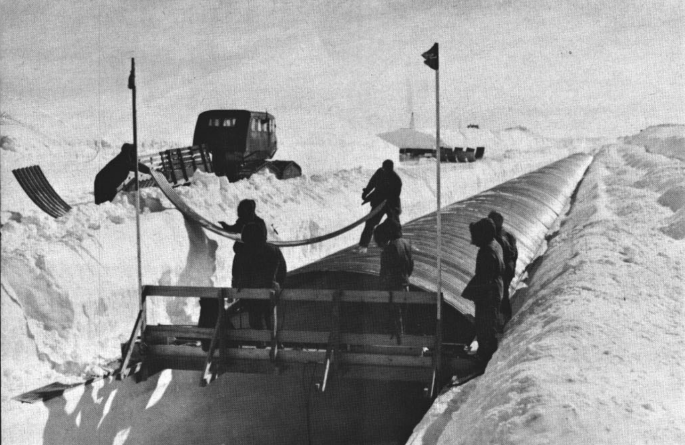
IN THE HOLE—Seabees place steel archways over snow tunnel that will house buildings at future Byrd Station.
