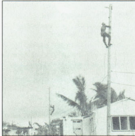
Seabees climb utility poles in a local Samoan village to help restore electrical power to the island.
