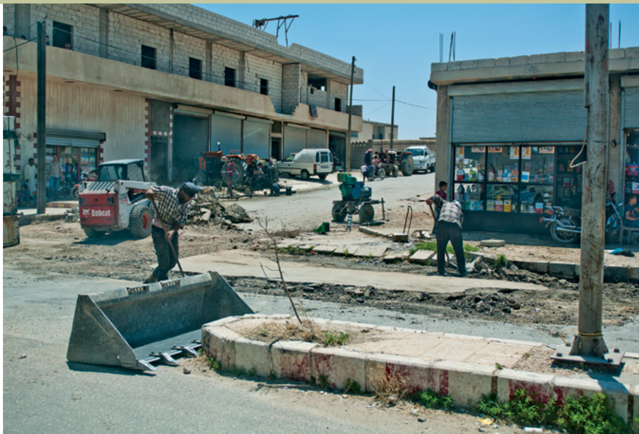
Men repair a road in a village outside Manbij, Syria. (U.S. Army photo)
