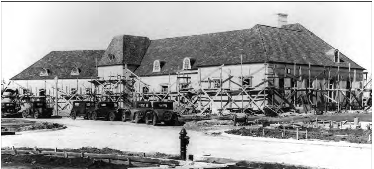
The Maxwell Field Officers Club, shown under construction in 1932, continued the same French Provincial style of the neighboring officer housing. In 2012 the club became an all-ranks club in response to declining membership and participation in both the officers and enlisted clubs at Maxwell.
