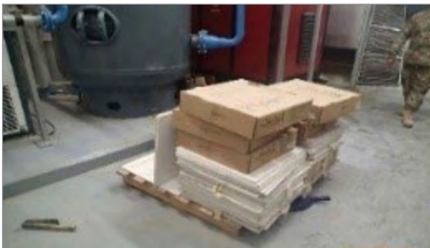
Storage of combustible material in mechanical room
