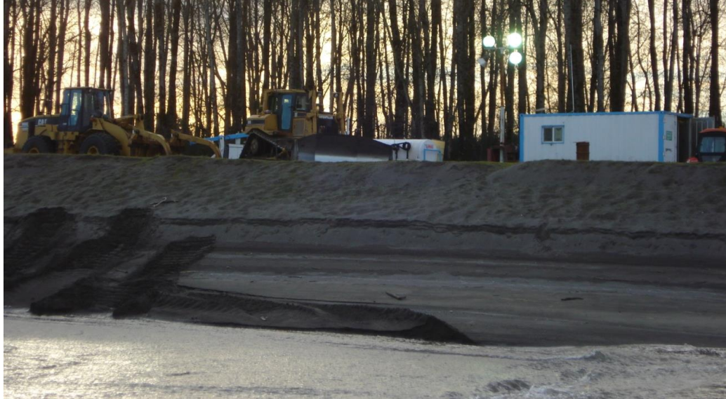
Figure 7 Staging equipment on top of the bank at Sand Island beach nourishment site
